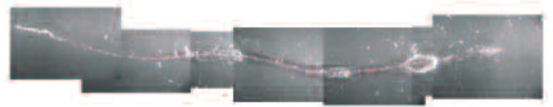
Cracked tube internal view
