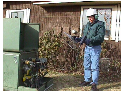
Figure 2-4 Technician Using Waveform Concentrator to Detect Ultrasonic Emissions from Underground Pad- mount Transformer
