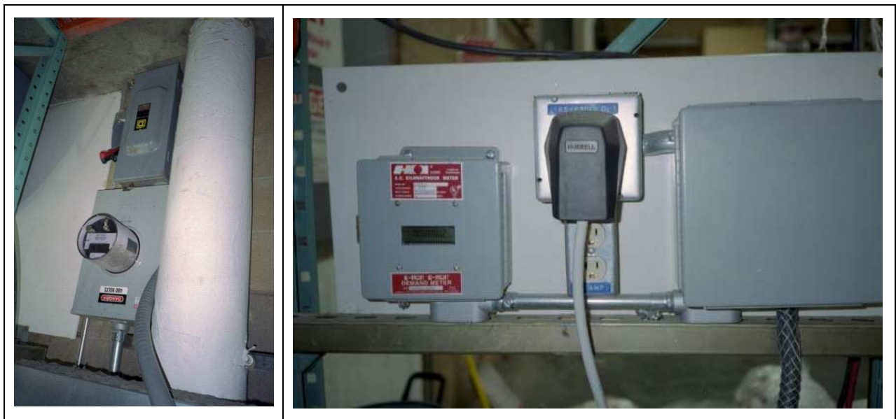
Figure 4-3 MLGW High-Power Charging Circuit Meter and Tennant Company Sub-Meter Panel
