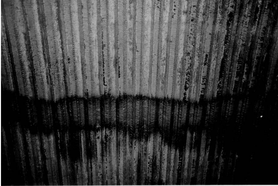
Figure 5-1 View of overlay after 5 months of service
