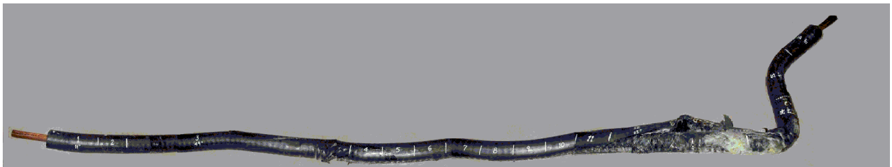
Figure 6-5 A Composite Photograph of the Damaged Cable
