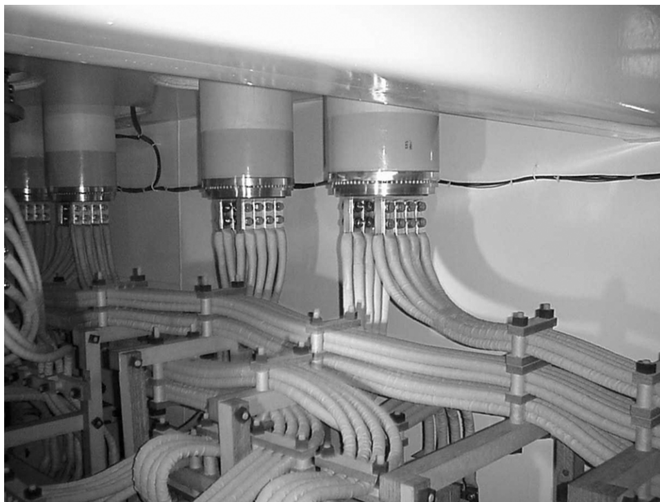
Figure 3-22 Flexible Connections between Transformer Winding and Bushings (Courtesy of Bob Beavers—Exelon)
