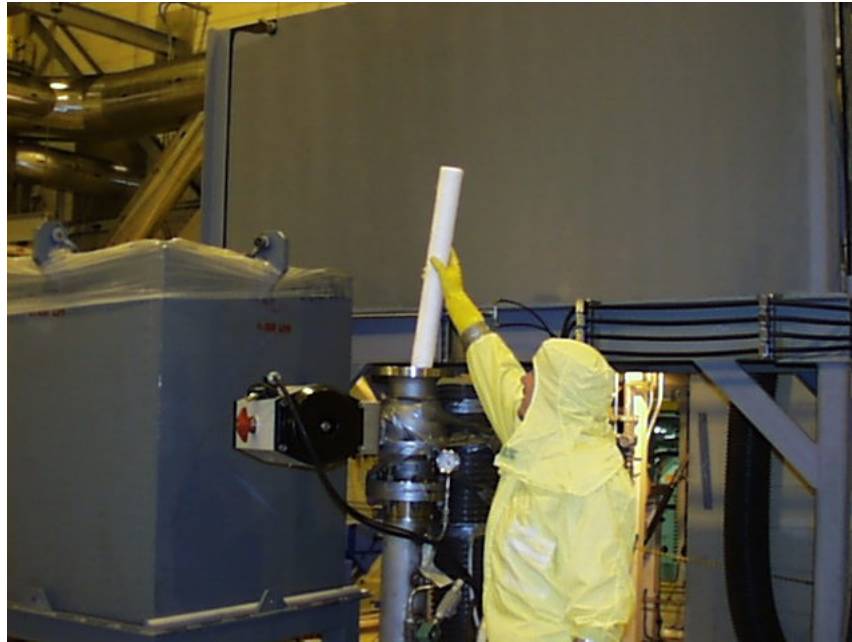
Figure 3-1 Manual Loading Of Filter Cartridge Into Tank Conversion Reformer
