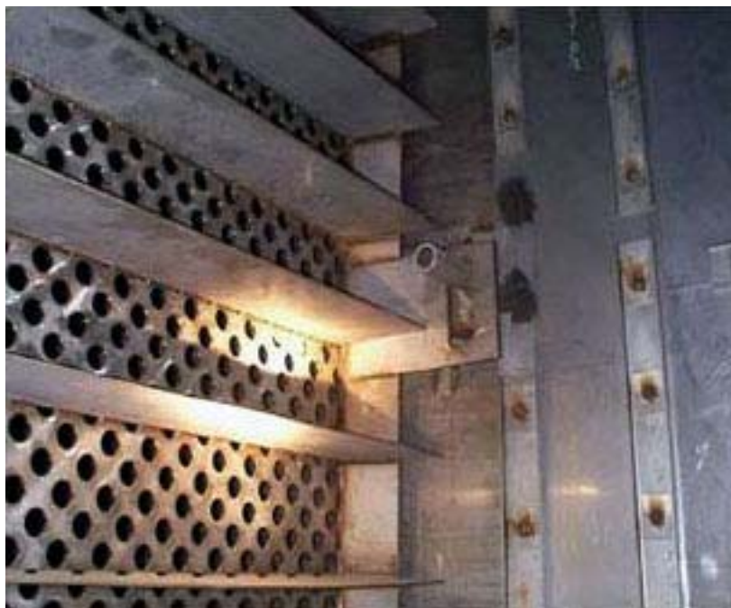
Figure 6-6 Flow straightening devices installed in HRSG.
