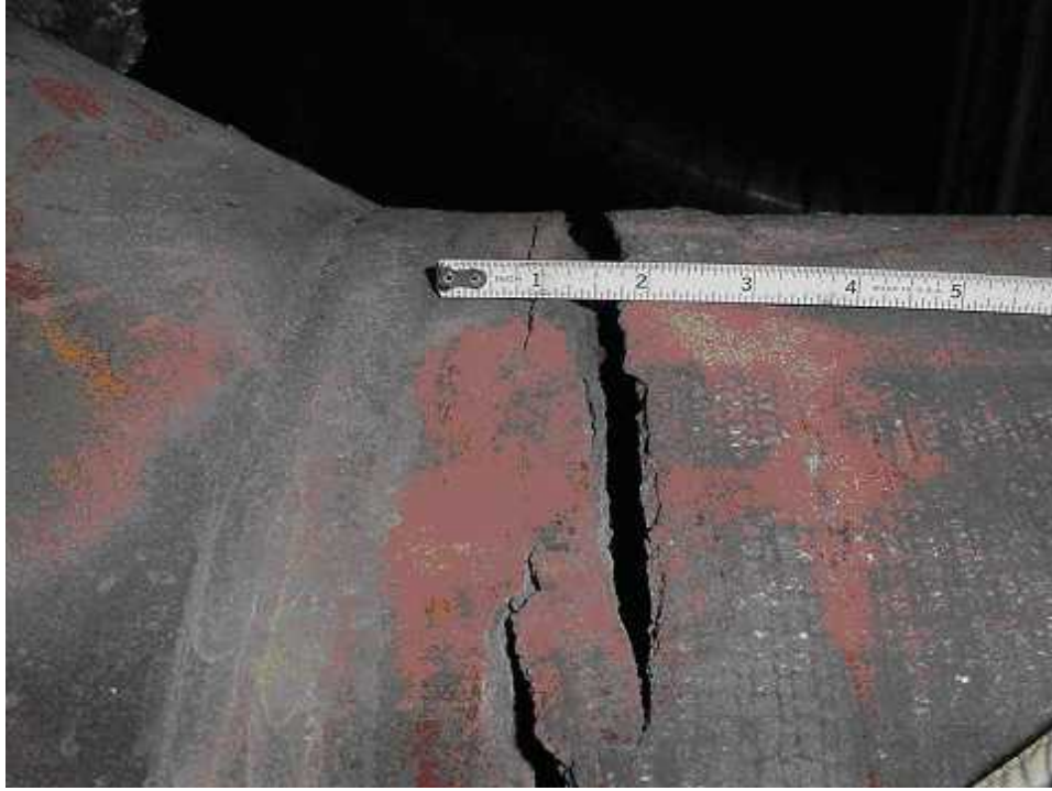
Figure 4-1 Girth Weld Damage in a SA 335, Grade 22 Main Steam Pipe Section at Gaston 5.
