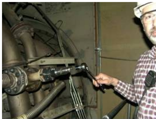
Figure 6-15 One of Fourteen Manual Values for Adjusting Secondary Fuel Flow to an Individual Combustor
