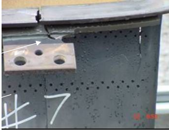
Figure 6-3 Complete Failure of Transition Piece and Evidence of Excessive Metal Temperature
