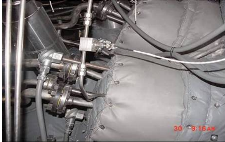
Figure 2-5 CD Sensor Installation on 501F
