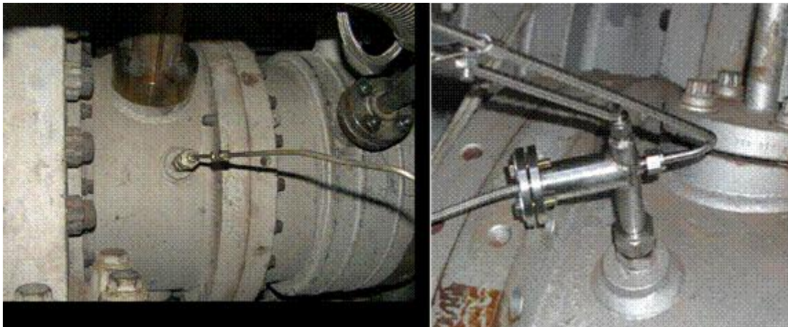
Figure 2-4 Installation of Transfer Tube for Low-Temperature Sensor (on the left) and Installation of a High-Temperature Sensor on GE Combustors
