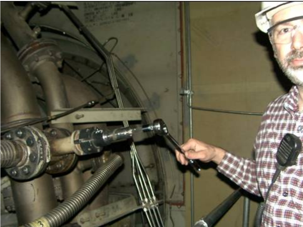
Figure 3-14 Manual Adjustments to Secondary Fuel Flow to Affected Combustor Can
