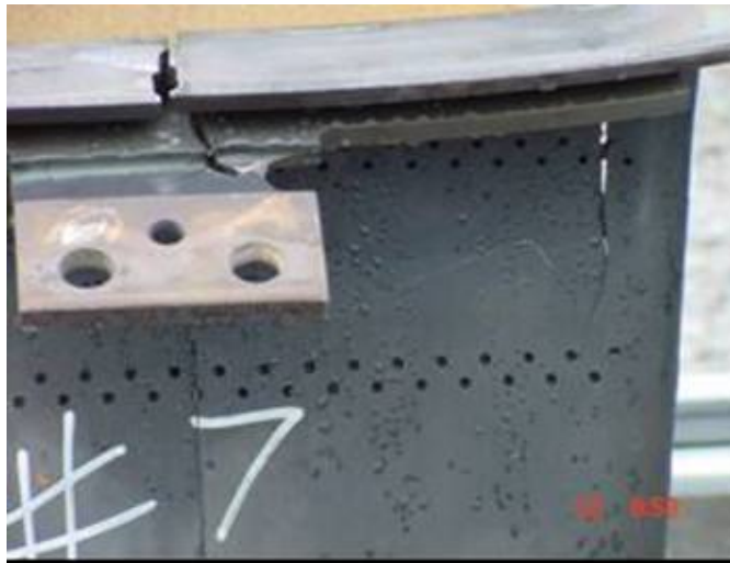
Figure 1-5 Complete Failure of Transition Piece and Evidence of Excessive Metal Temperature
