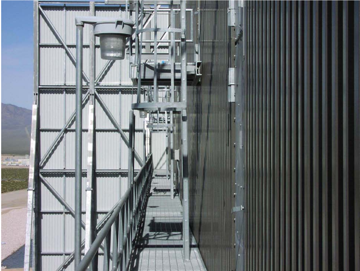
Figure 4-5 External Walkway and Caged Ladder on a Typical Air-Cooled Condenser
