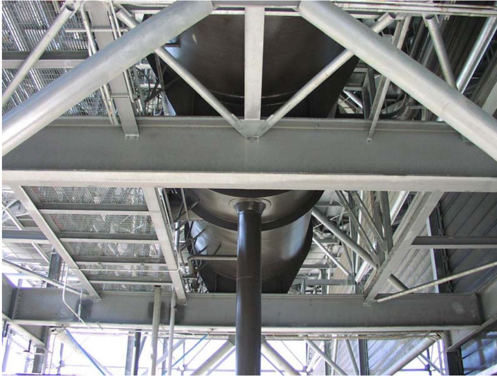
Figure 4-3 Example Condensate Tank, Piping, and Access
