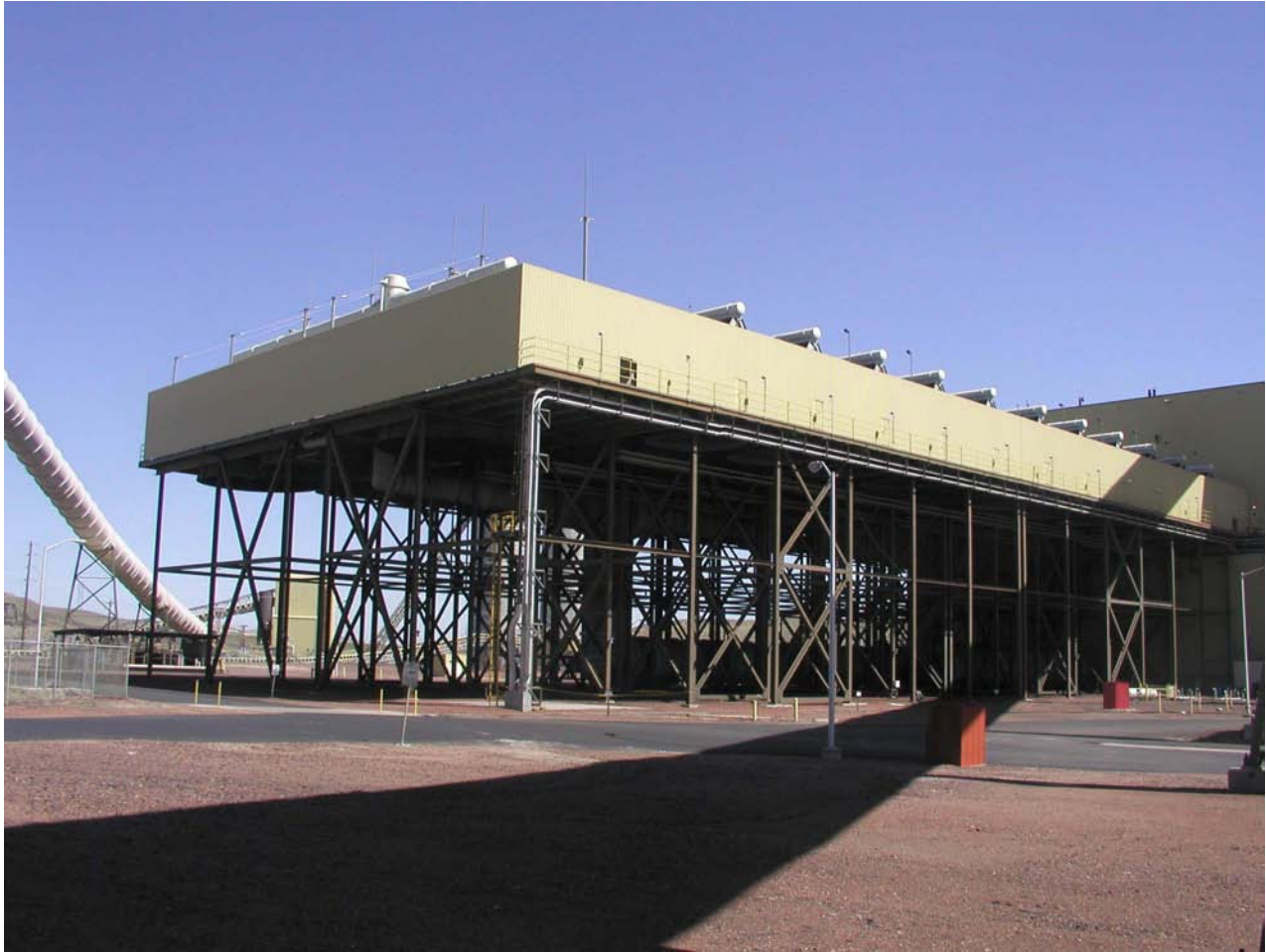
Figure 2-5 Wyodak Air-Cooled Condenser
