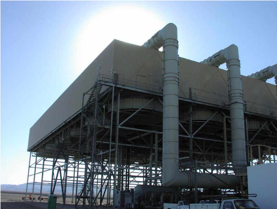
Figure 2-4 Air-Cooled Condenser at El Dorado Generating Station – Depicting 3 of 5 Streets
