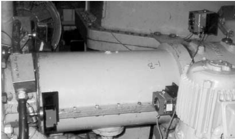
Figure 2-2 Coupling Cover for Continuous-Lubricated Coupling Courtesy Rota-Tech Inc.
