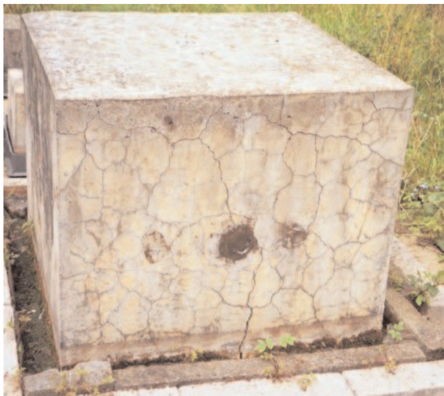
Figure 1. ASR Damage to Concrete Mixture Using a Reactive Aggregate with Portland Cement (Courtesy of Thomas, et al. , University of Toronto)
