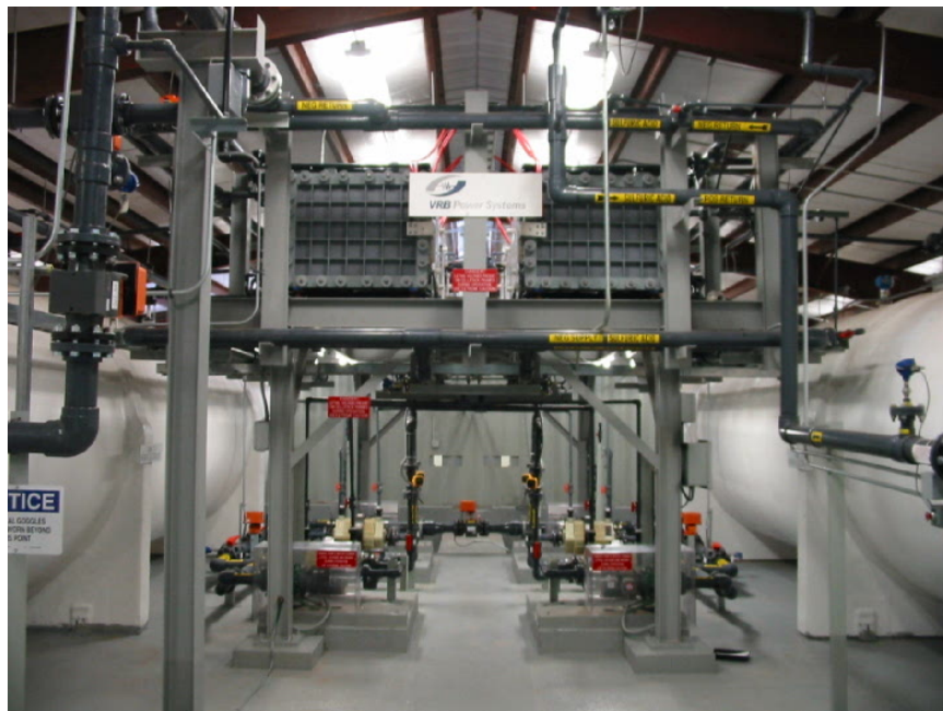
Figure 3-8 VRB Battery at Moab, Utah
