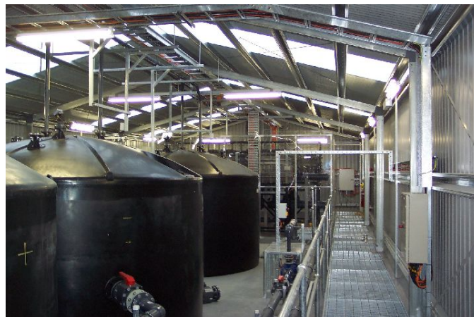
Figure 4-1 VRB Facility on King Island, Tasmania (Courtesy HydroTasmania and Pinnacle VRB)
