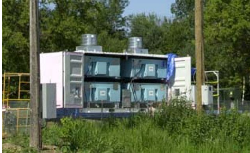
Figure 3-9 Zinc-Bromine Battery Installation at Lum, Michigan (Courtesy ZBB Energy Corporation)
