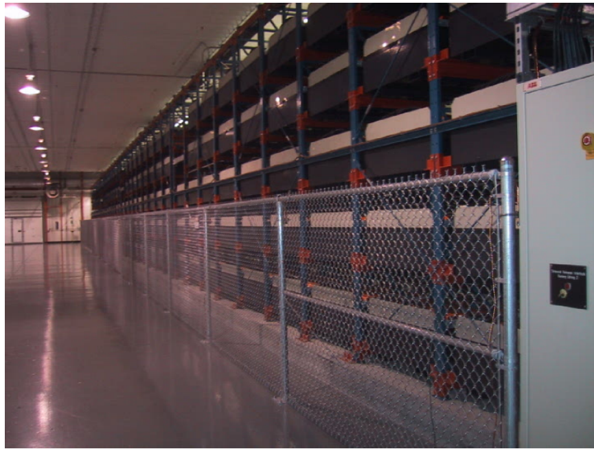
Figure 3-5 Battery Banks From the GVEA BESS
