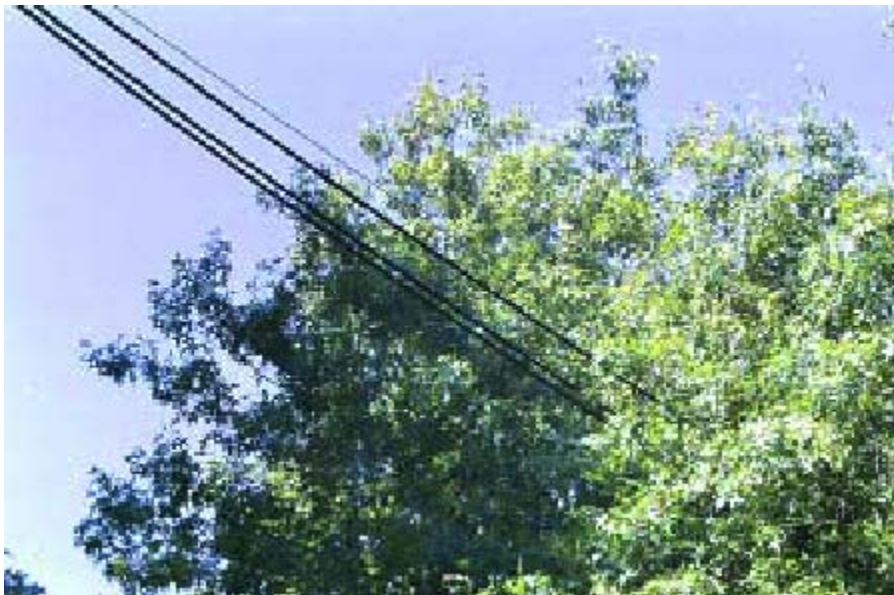
Figure 3-2 Example of a Spacer Cable Run Through Trees
