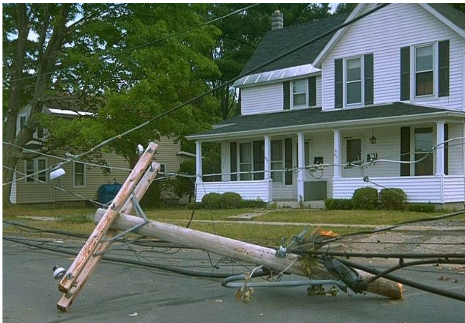
Figure ES-1 A Pole Broken in Half by a Tree Falling onto the Line Structure During a Windstorm
