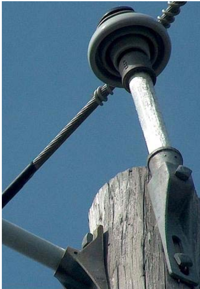
Figure 6-6 Vertically Mounted Fiberglass Standoff Bracket Showing Surface Degradation
