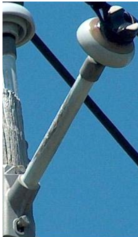
Figure 6-8 Fiberglass Standoff Bracket Showing Surface Degradation
