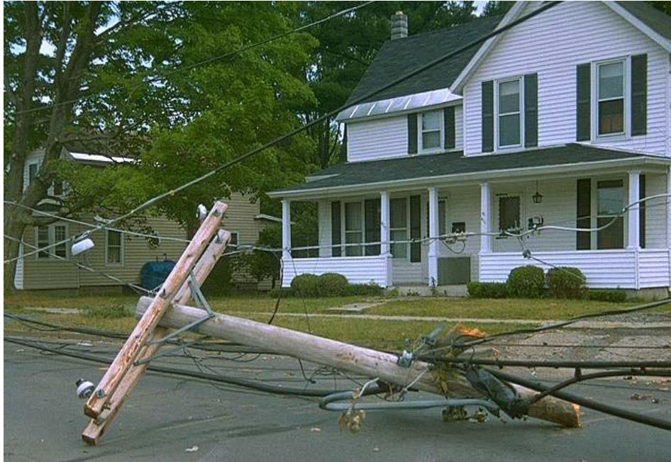
Figure 3-10 A Pole Broken in Half by a Tree Falling Onto the Line Structure During a Windstorm
