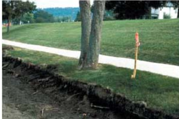
Figure 4-11 Example of Root Damage due to Excavation
