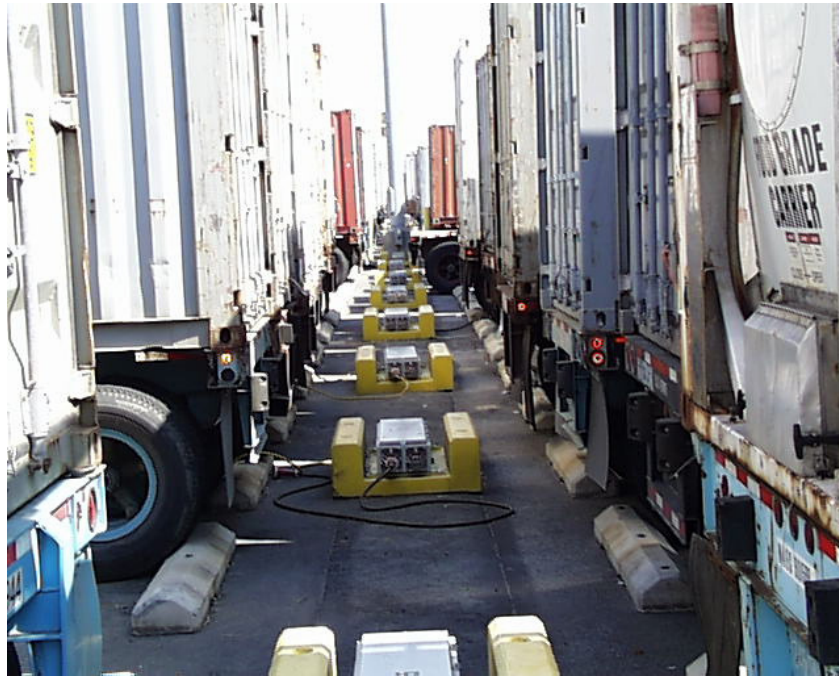
Figure 1-1 Container Refrigeration systems plugged in at port
