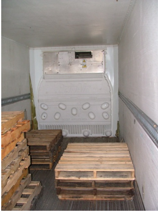
Figure 3-2 Evaporator Side of a TRU
