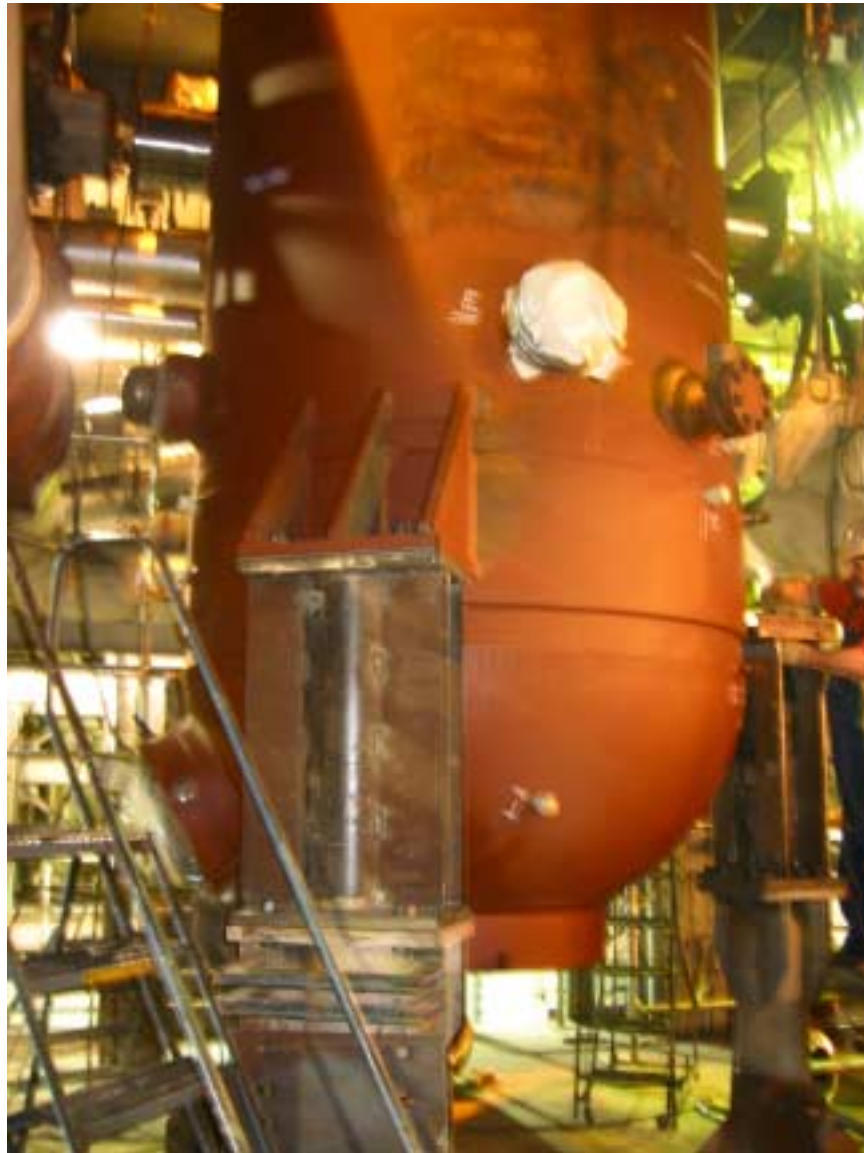
Figure 3 New Feedwater Heater Showing Support Leg Extensions
