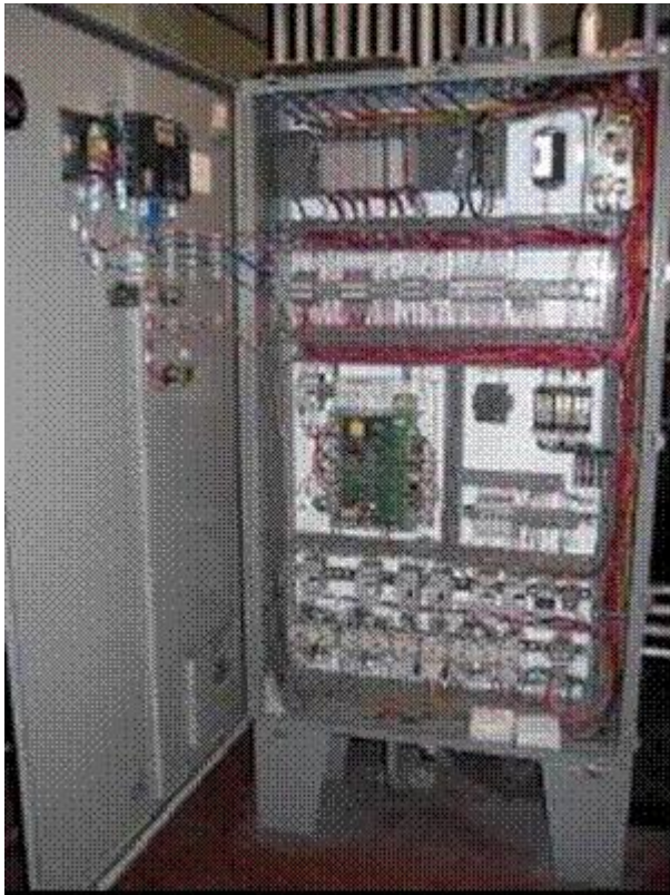
Figure 2-10 Primary Control Panel
