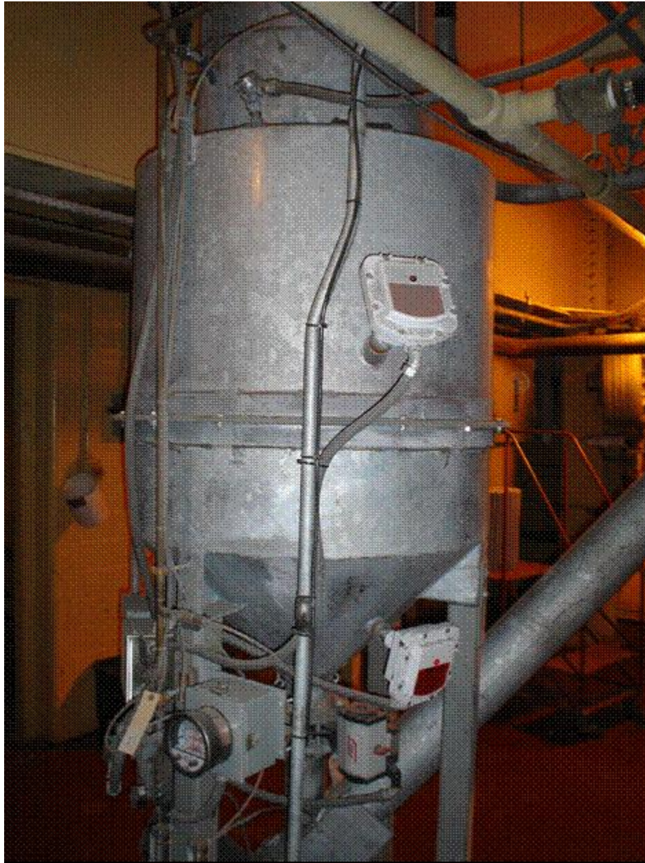
Figure 2-7 Calcium Hypochlorite Day Storage Bin
