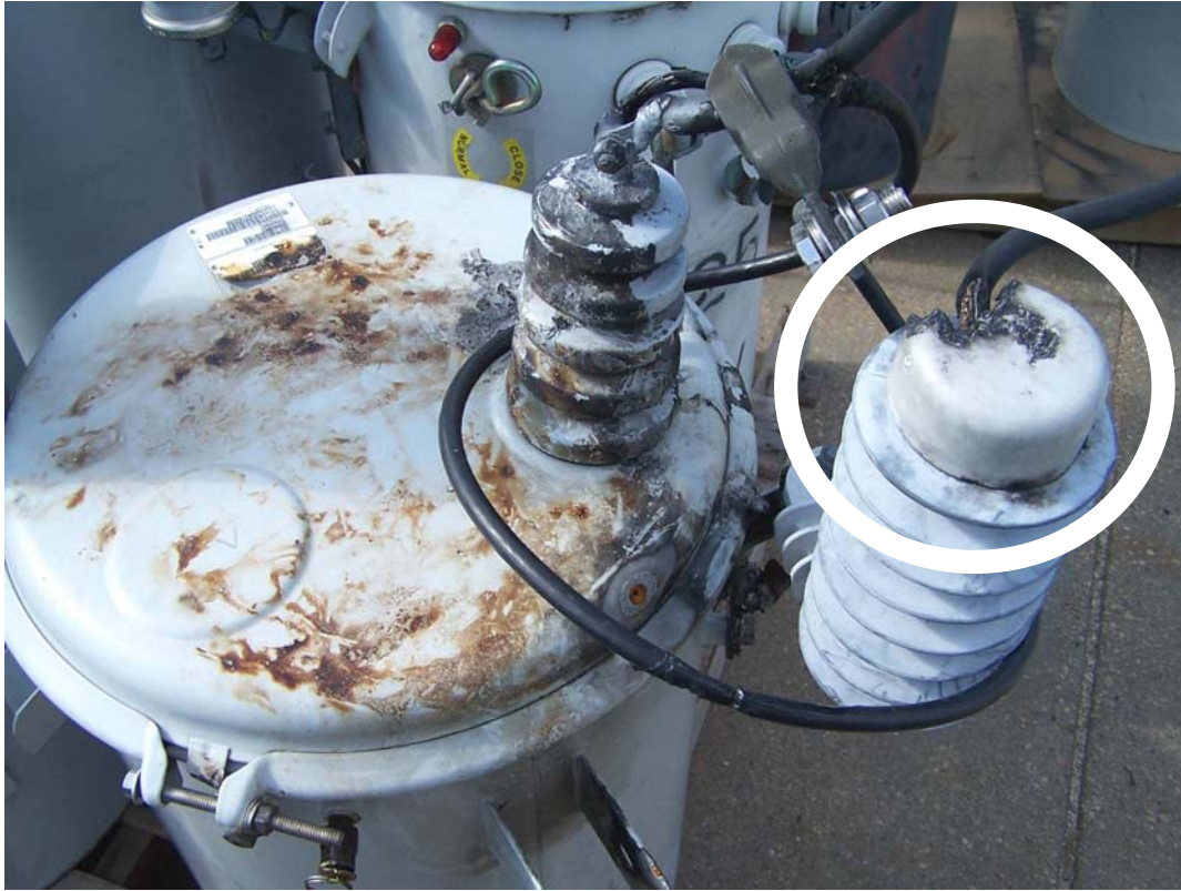
Figure 4-18 Transformer with Failed Tap
