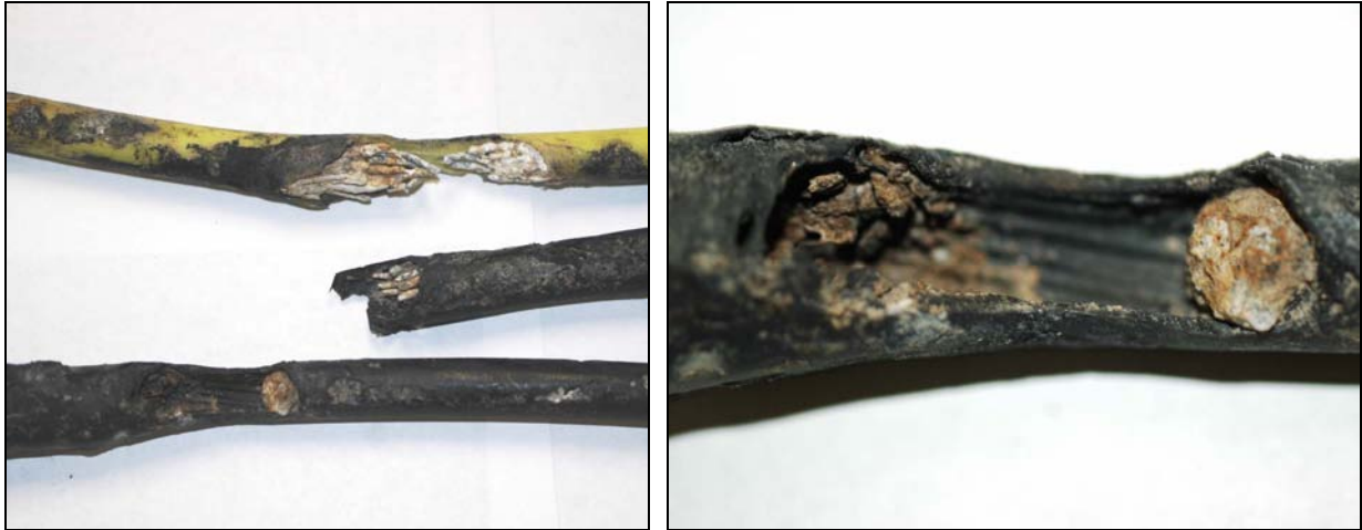
Figure 4-13 Deteriorated and Corroded Cables Responsible for Intermittent Arcing and Outages
