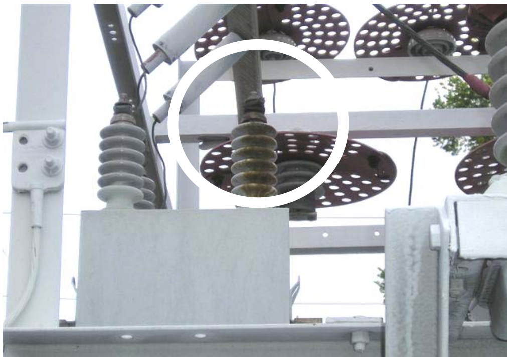
Figure 4-20 Substation Bus Capacitor with Failing Bushing
