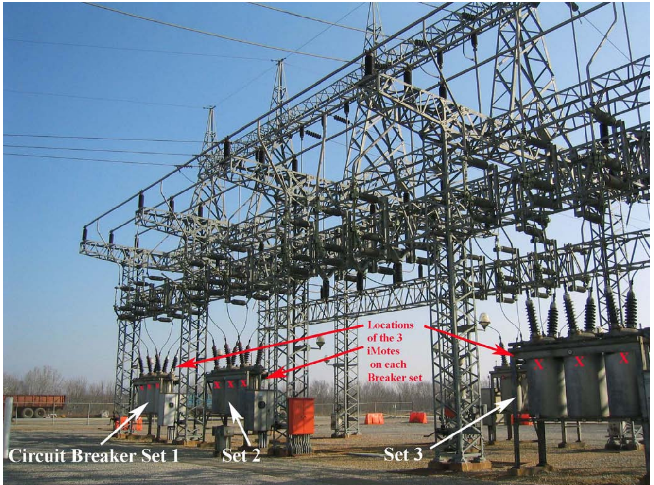
Figure 4-6 Location of the sensors on the breakers at TVA
