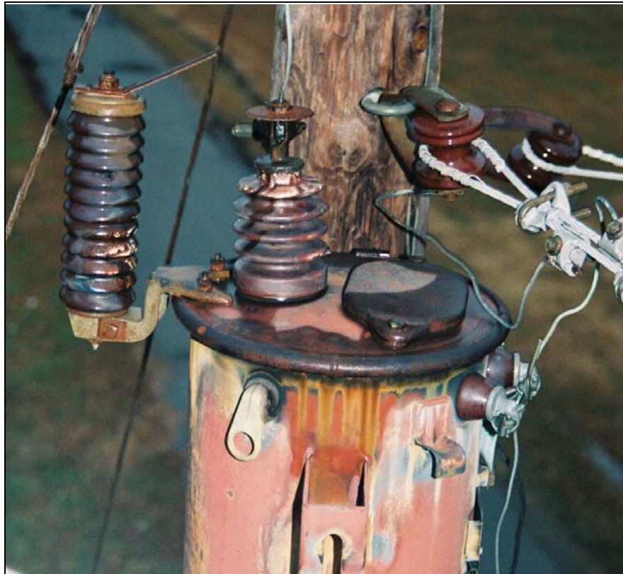
Figure 3-5 Poletop Transformer with Damaged Bushing That Caused Intermittent Faults
