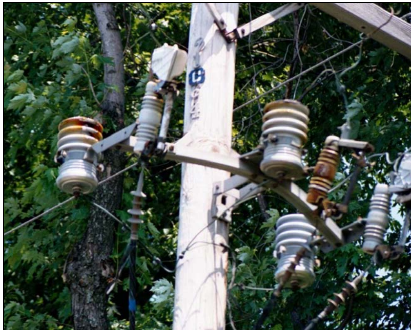
Figure 5-2 Riser-Pole Installation With Evidence of Multiple Arc Burns
