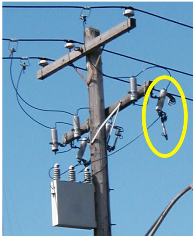
Figure 9-3 Overhead Distribution Capacitor Installation with Blown Fuse
