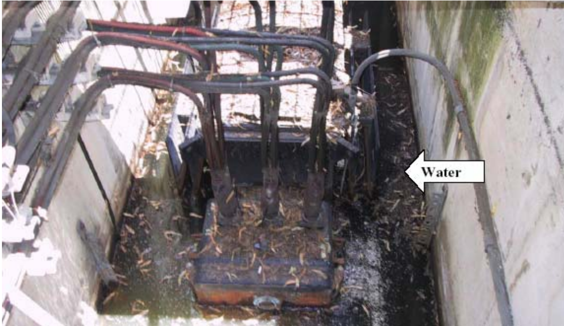
Figure 2-17 Flooded Transformer Vault with Floating Debris Source: (Stone & Webster Consultants 2001)
