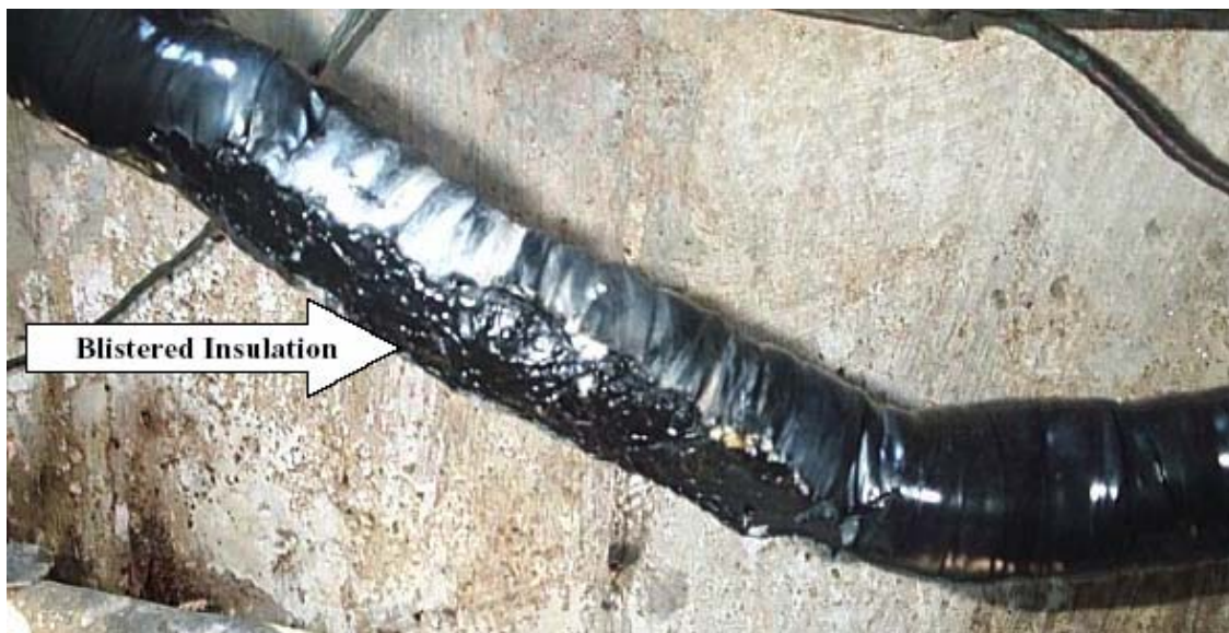
Figure 2-20 Secondary Splice with Visible Signs of Overheating Source: (Stone & Webster Consultants 2001)
