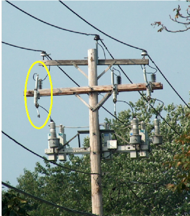
Figure 9-4 Fuse Tubes Should Not be Left Hanging Upside Down
