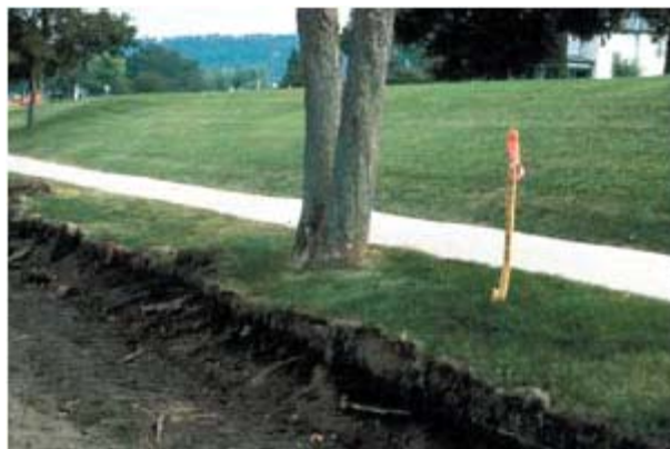
Figure 6-8 Example of Root Damage Due to Excavation
