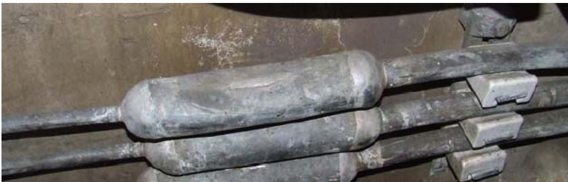
Figure 2-18 Partially Imploded Cable Splice
