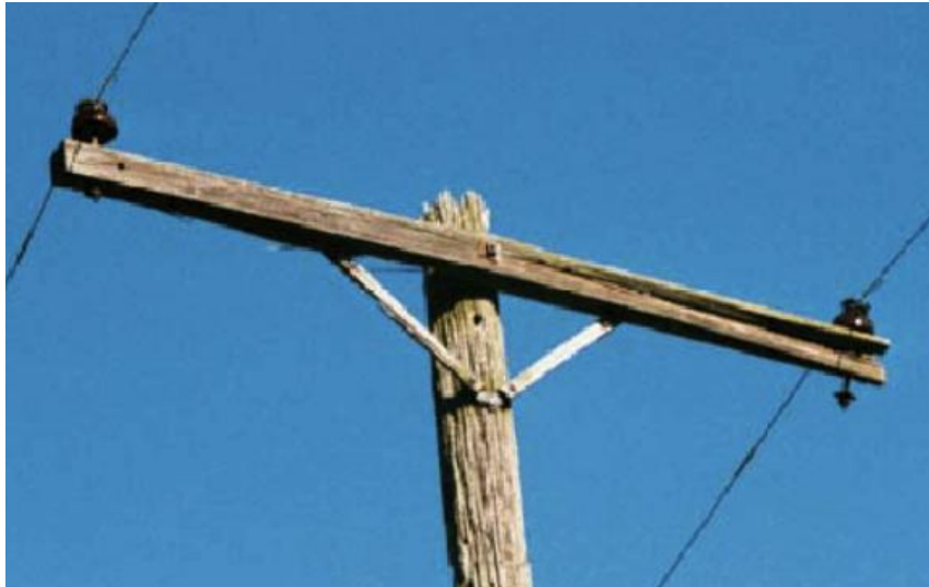
Figure 2-8 Broken / Split Crossarm and Pole Showing Signs of Shell Rot
