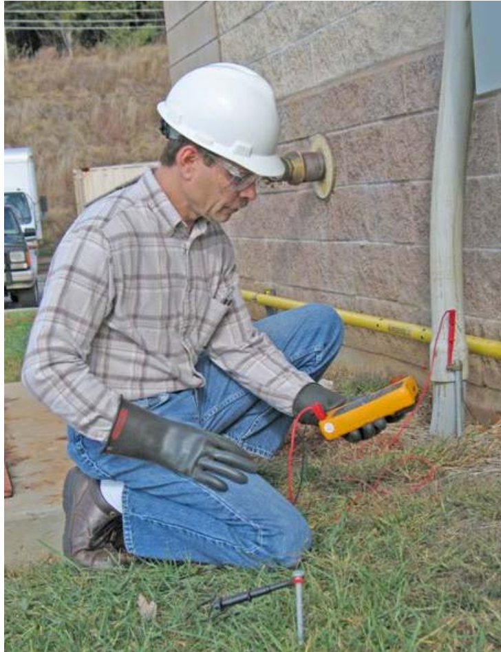
Figure 7-11 Sample Measurements Between a Grounded Meter Base and a Reference Ground
