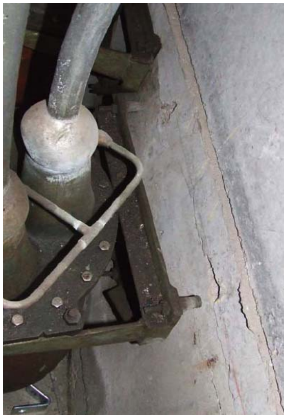
Figure 2-24 Y-Bucket That Has Pulled Away From Support
