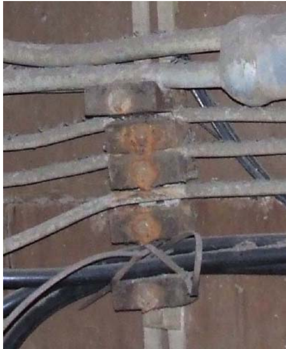
Figure 2-23 Wood-Block Supports in Various Stages of Decay
