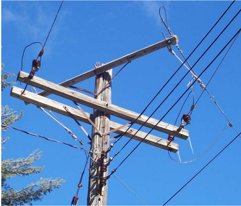
Figure 2-14 Hastily Repaired Storm Damage Should be Identified During a Visual Inspection
