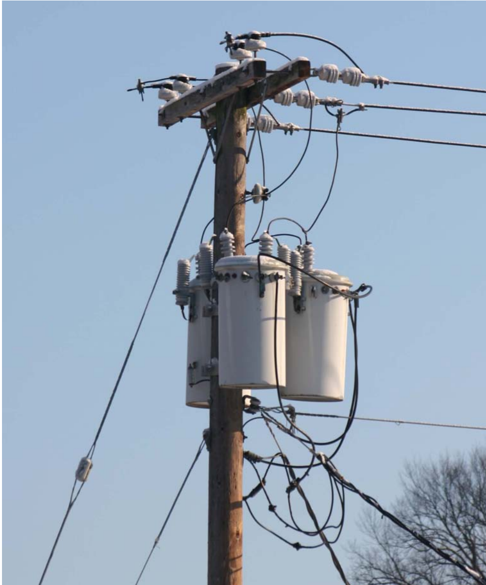
Figure 5-5 Distribution Structure with Multiple Deficiencies – No Local Fuses, No Animal Guards, and Poor Clearances
