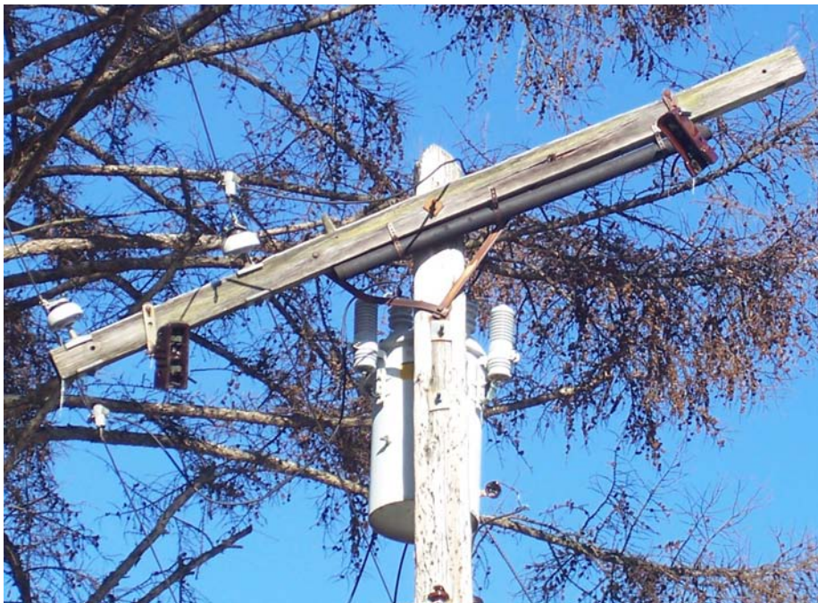
Figure 2-9 Partially Detached Crossarm and Bent Crossarm Brace Note the metal pipe strapped to the underside of the crossarm. At the time of writing the purpose of this pipe was not clear
