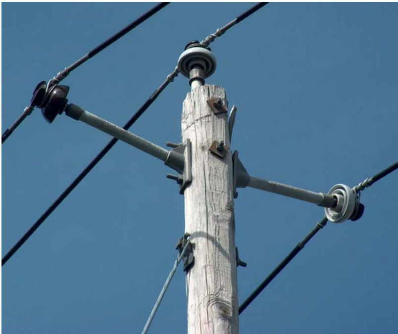
Figure 2-7 This Pole Top Appears to be Splitting and Allowing the Insulator Standoff to Pull-Away. (Also notice the heavy surface degradation on the insulator standoffs)
