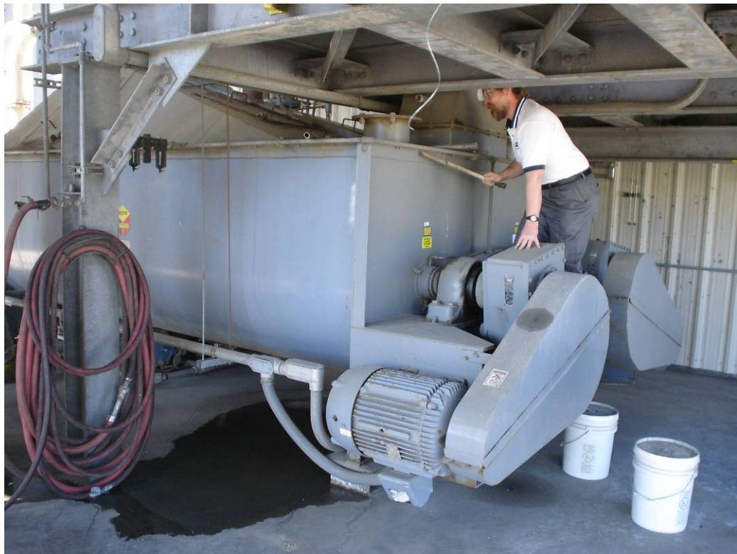
Figure 3-6 Low Speed Mixer – Inlet Side
