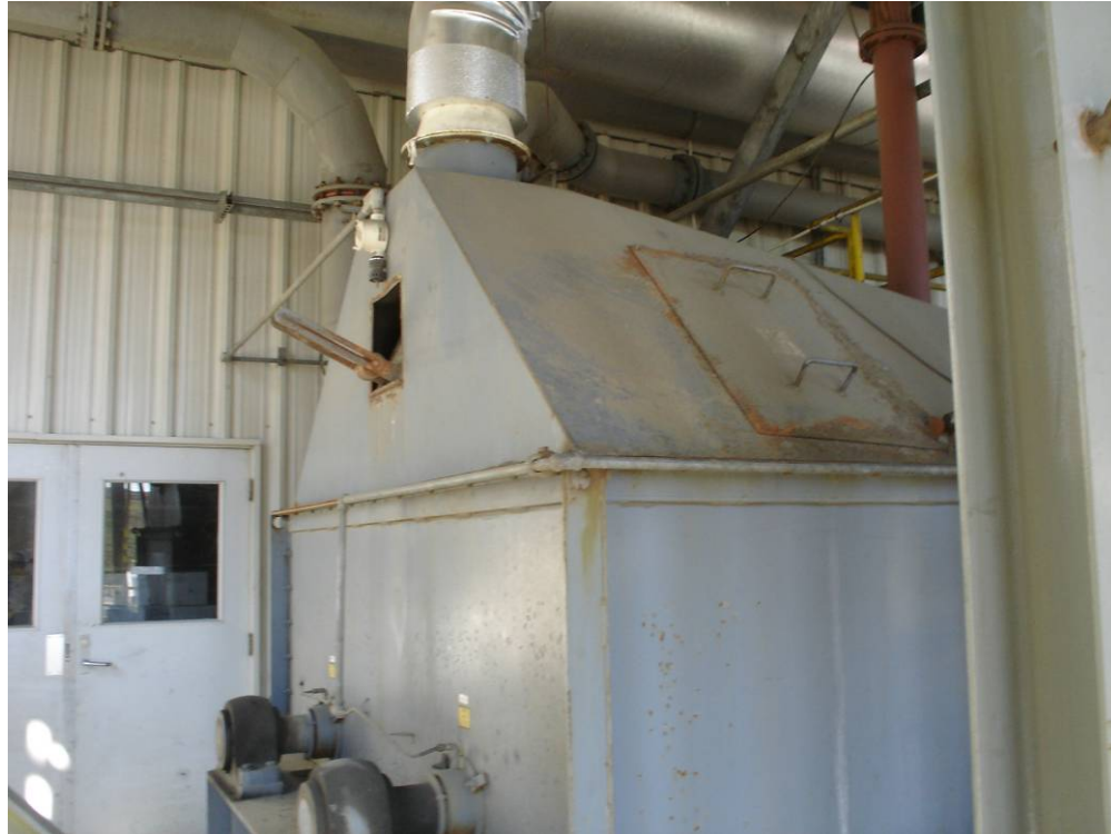
Figure 3-7 Low Speed Mixer – Outlet Side
