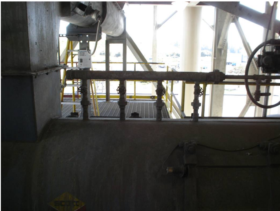
Figure 3-5 Detailed Mixer View Showing Water Injection Piping (4 lines)
