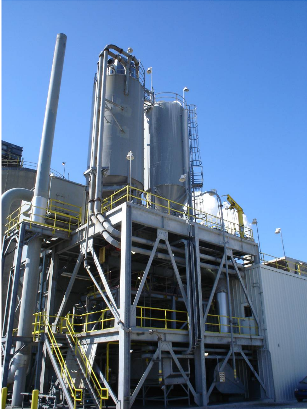
Figure 3-1 Ammonia Removal Processing Area
