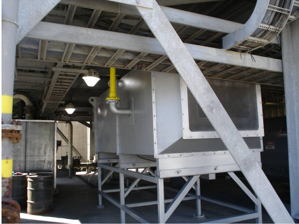
Figure 3-8 Natural Gas Burner for Dryer
