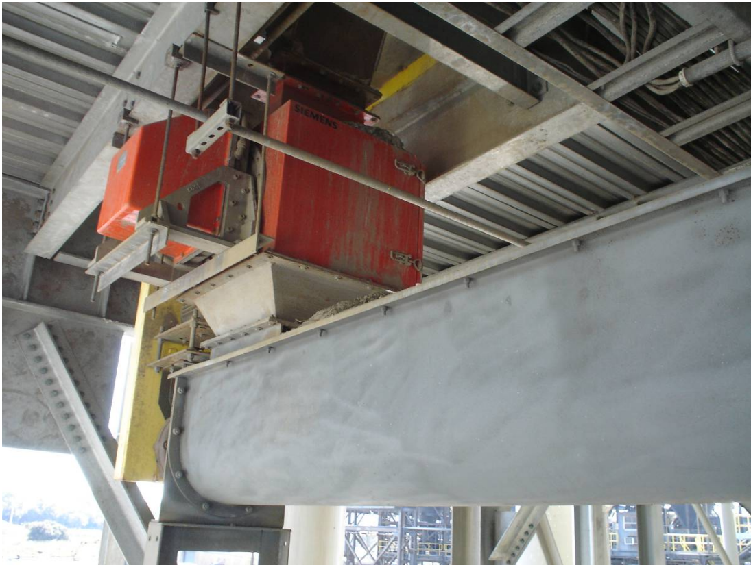
Figure 3-2 Ash Metering and Screw Transport
