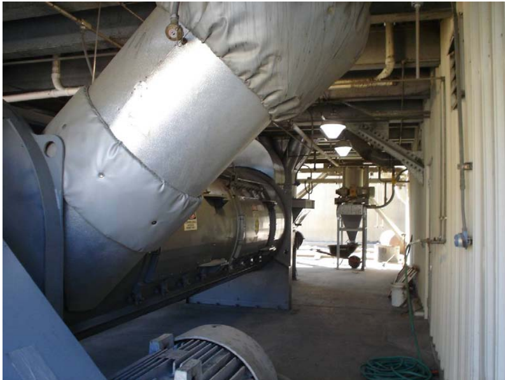
Figure 3-9 Air-Swept Tubular Dryer
