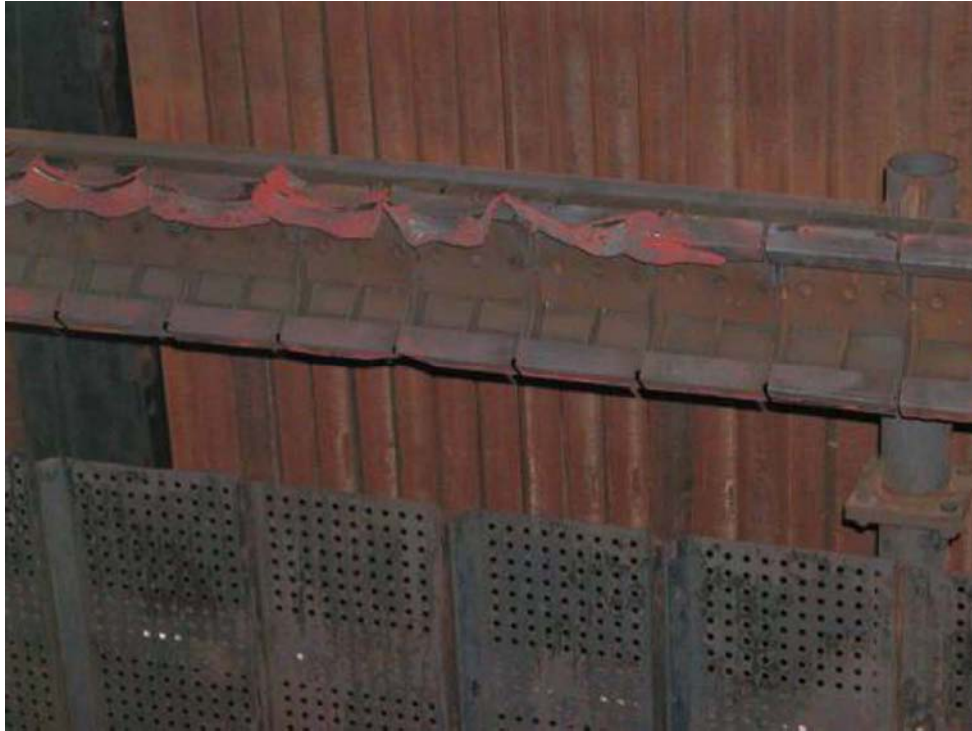
Figure B-2 Close Up of Duct Burner Damage
