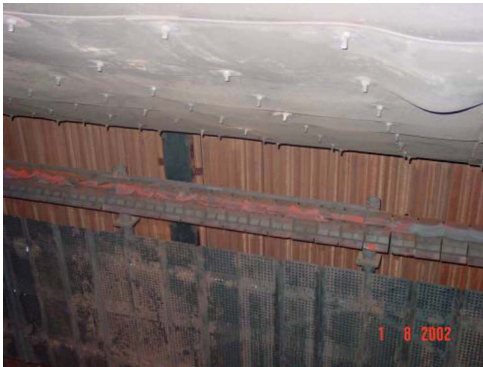
Figure B-1 Damage to Duct Burner Assembly and Firing Duct Stainless Steel Liner above Duct Burner. Overheating damage (not shown in photo) also occurred in the HRSG outer casing adjacent to locations where liner damage was most severe.
