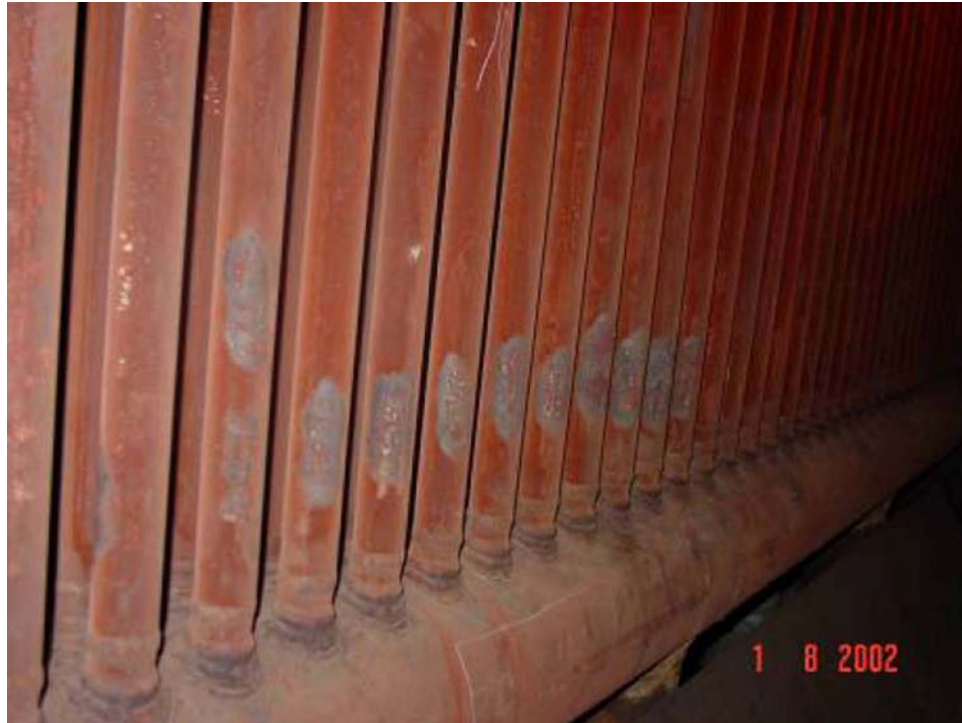
Figure B-3 Visible Evidence (Oxide Spalling) on First Row of Superheater Tubes (Unfinned) Downstream of Duct Burner
