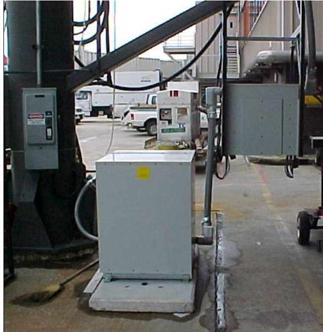
Figure 2-4 Power server (I) and station (above)
