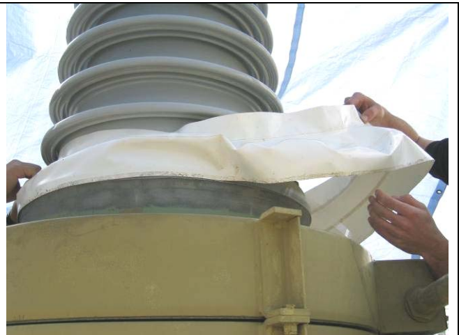
Step 2: Application of the inner flexible shell
