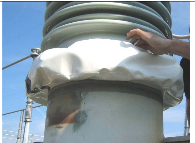
Step 2: Application of the inner flexible shell
