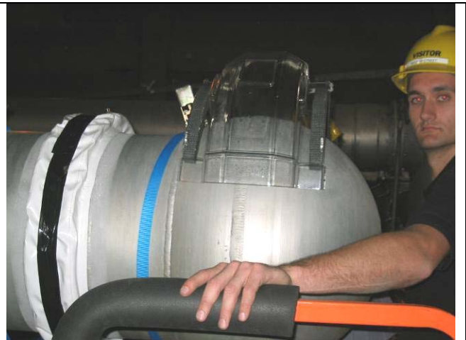
Step 2: Application of the inner flexible shell
