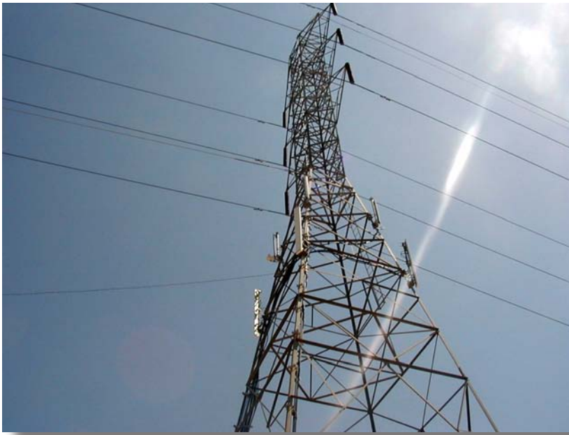
Figure 2. Mobile telecommunications antennas mounted on an electric power transmission tower.
