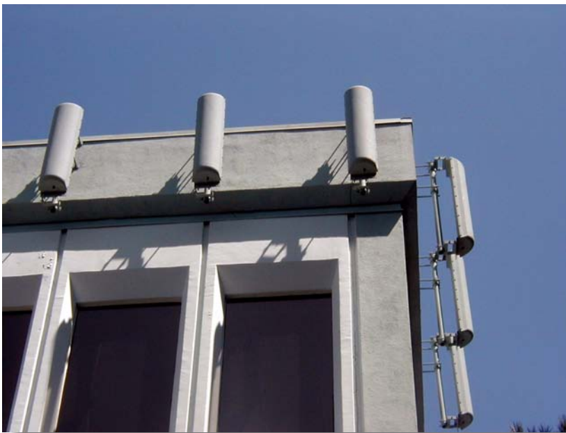
Figure 1. Mobile phone base station antennas on a building.
