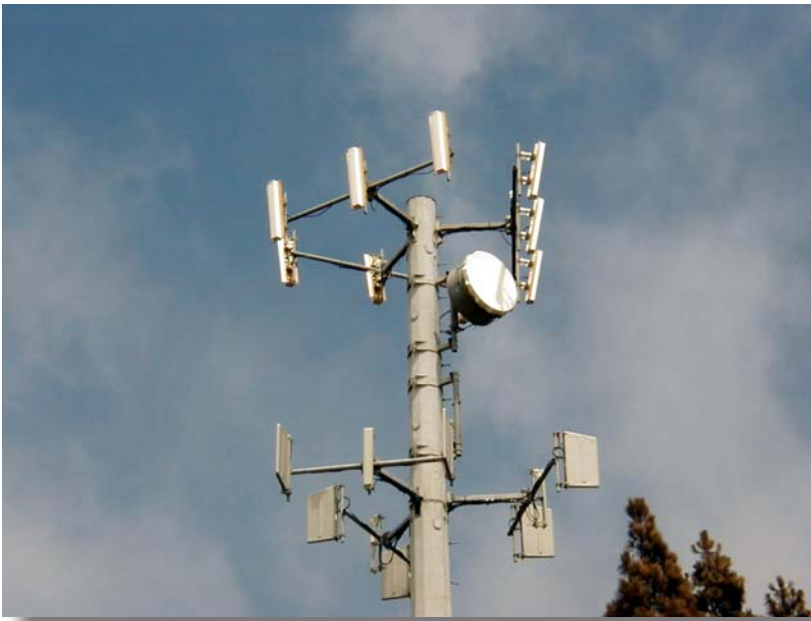
Figure 6. A mobile phone base station with an antenna array on a freestanding tower.
