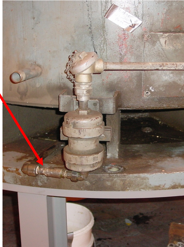
Figure 4-28 Lower Bearing Oil Level Switch
