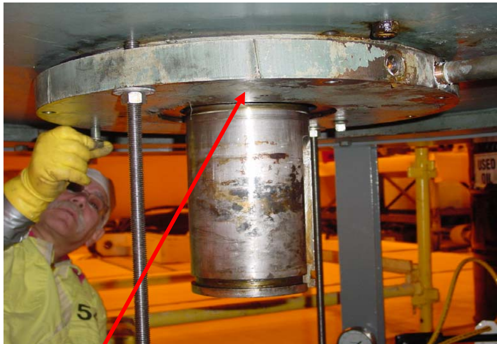
Figure 4-30 Lower Bearing Oil Pan Being Installed
