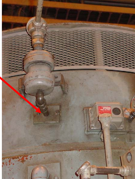
Figure 4-24 Upper Bearing Potential Leak Paths
