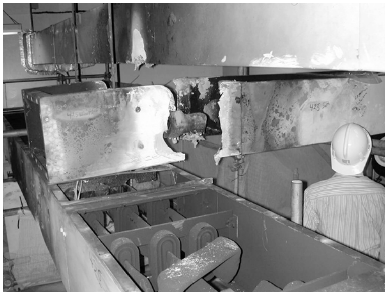
Figure 3-5 Diablo Canyon Bus Duct Damage
