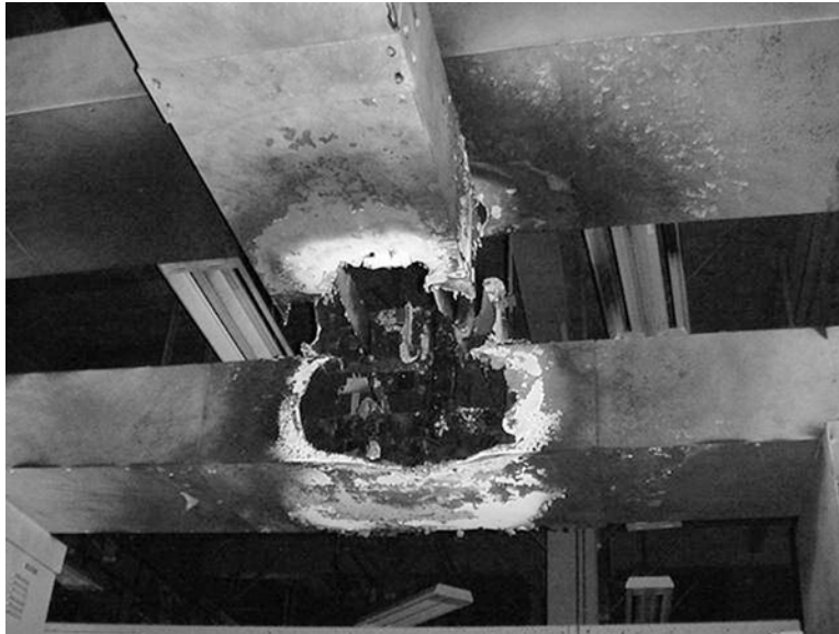
Figure 3-4 Diablo Canyon Bus Duct Damage
