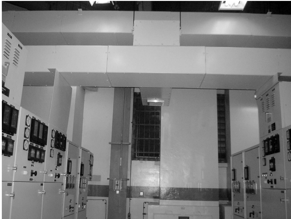
Figure 6-1 Diablo Canyon Bus Duct Repair
