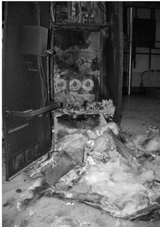
Figure 3-7 Prairie Island Switchgear Damage
