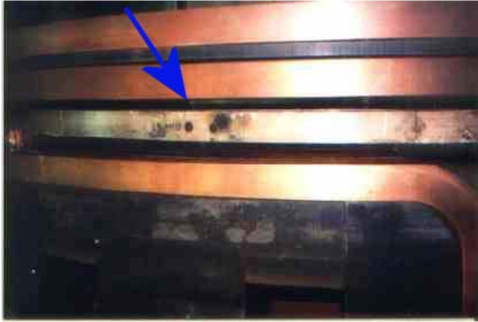
Figure 2-3 End Turn Arcing Damage
