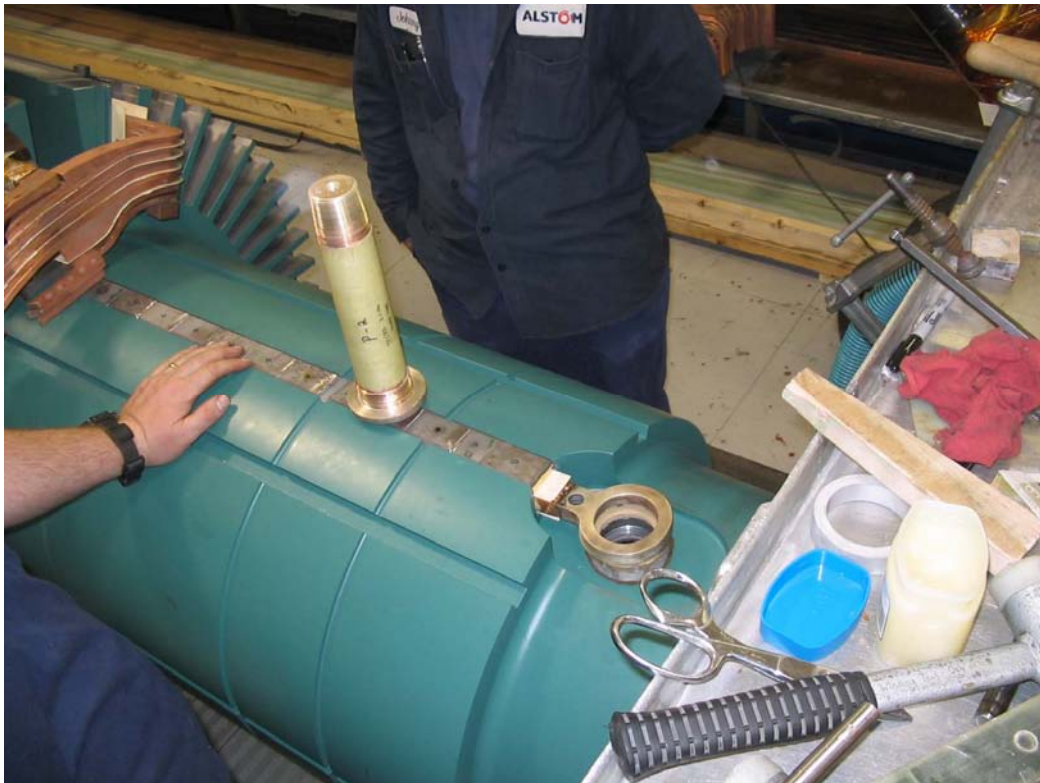
Figure 2-7 Radial Stud Removed from Shaft
