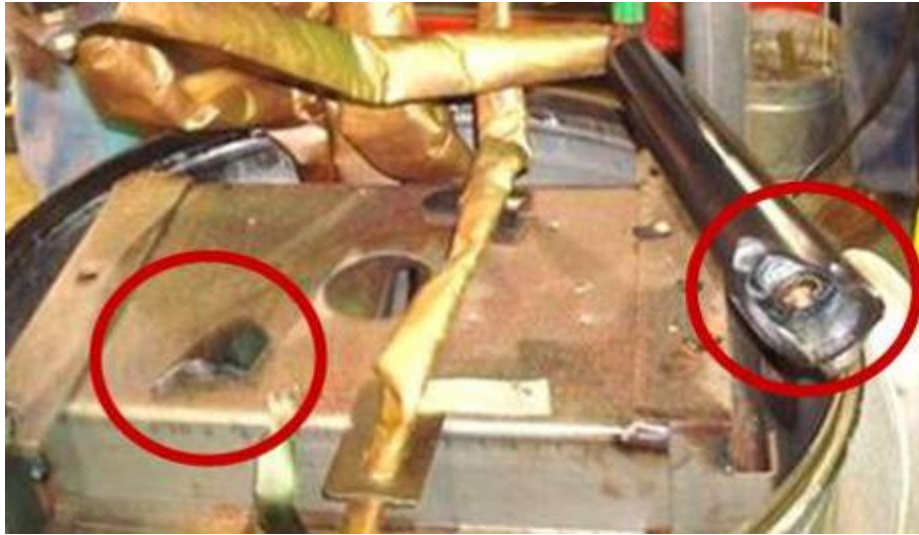
Figure 3-26 Failed Internal Transformer Bushing
