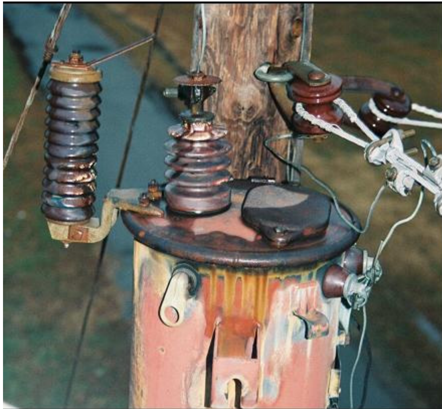
Figure 3-6 Transformer With Damaged External Bushing That Caused Intermittent Faults
