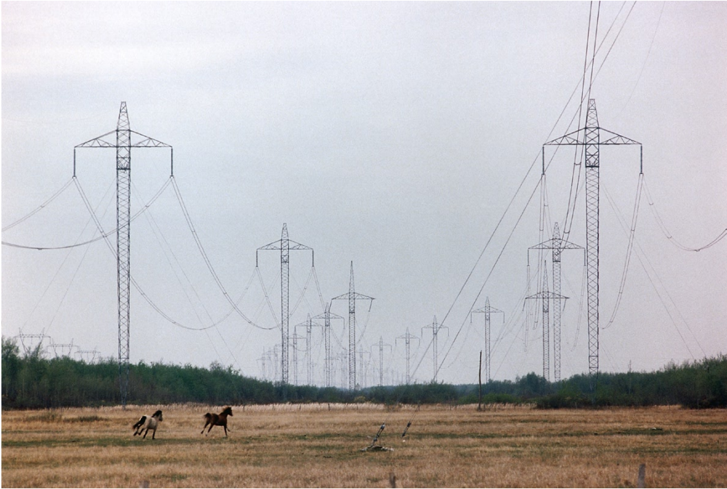
Figure 5-2 Nelson River HVDC Transmission Lines
