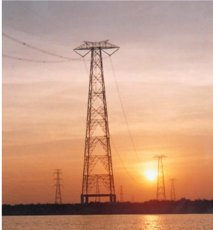
Figure 5-4 POWERGRID \pm 500 kV HVDC Line
