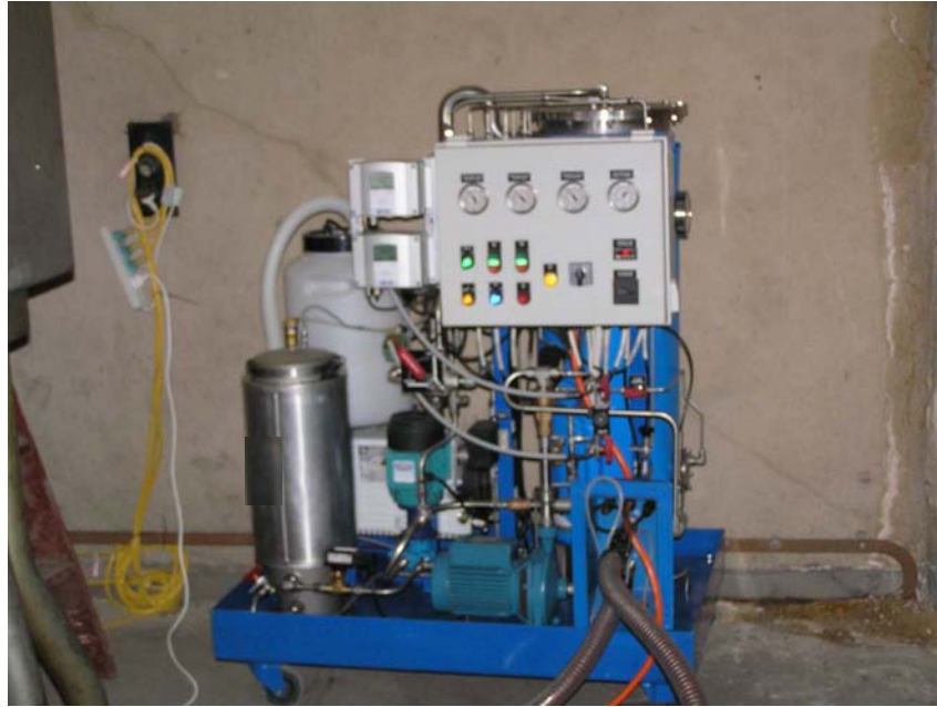
Figure 2-2 Vacuum On-line Dryout Unit in Operation
