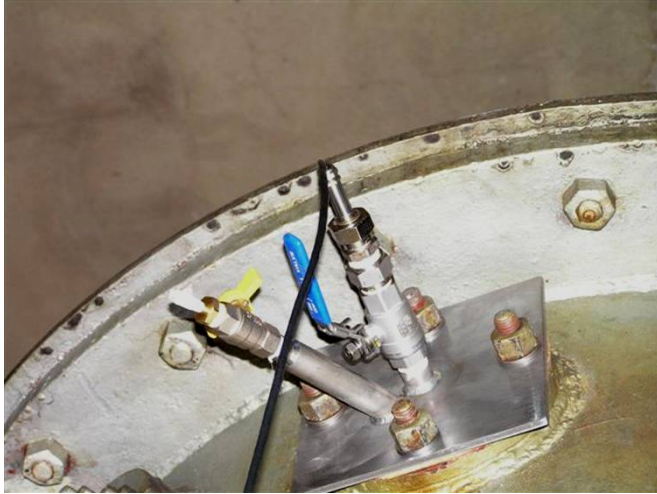
a) Top of Transformer
