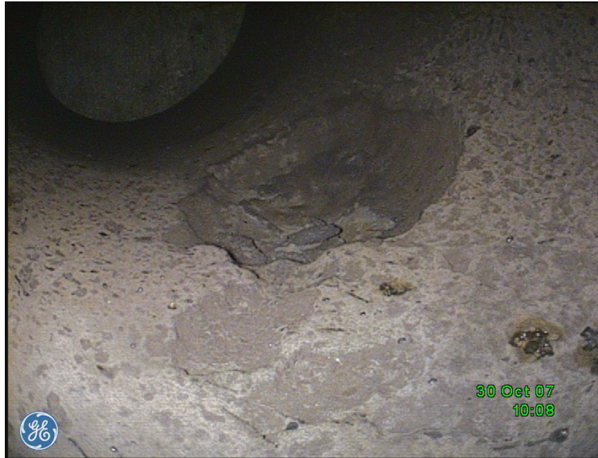
Figure 6-3 Localized Wall Loss in the Pit Seen in Figure 6-1 (Removal of the tube section would confirm the presence of hydrogen damage.)
