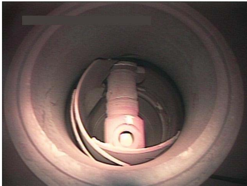
Figure 4-1 Desuperheater Nozzle with a Damaged Liner as Seen by RVI
