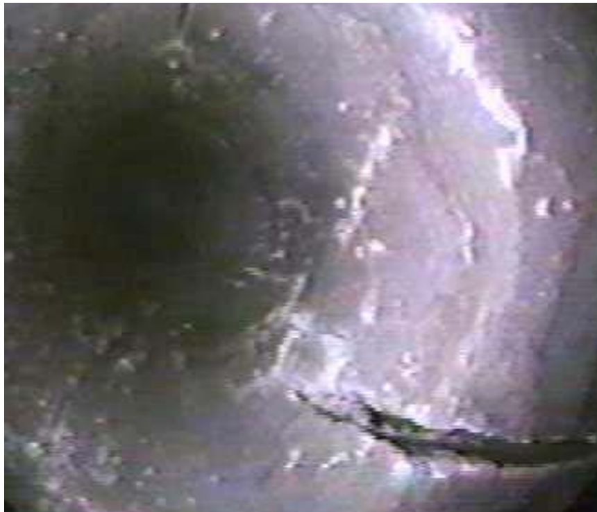
Figure 3-12 Crack in the Tube Wall as Documented with RVI
