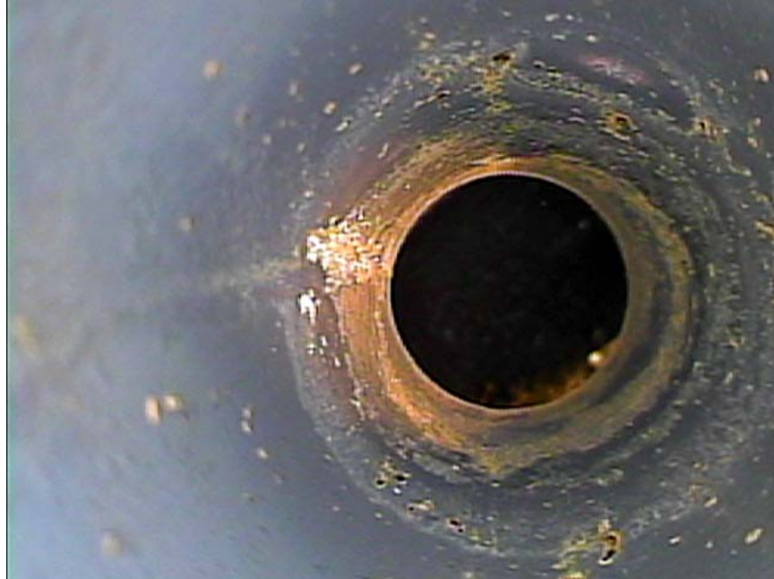
Figure 9-2 Flow-Accelerated Corrosion as Found by RVI in a Boiler Tube: This Damage Has Been the Cause of Tube Failures
