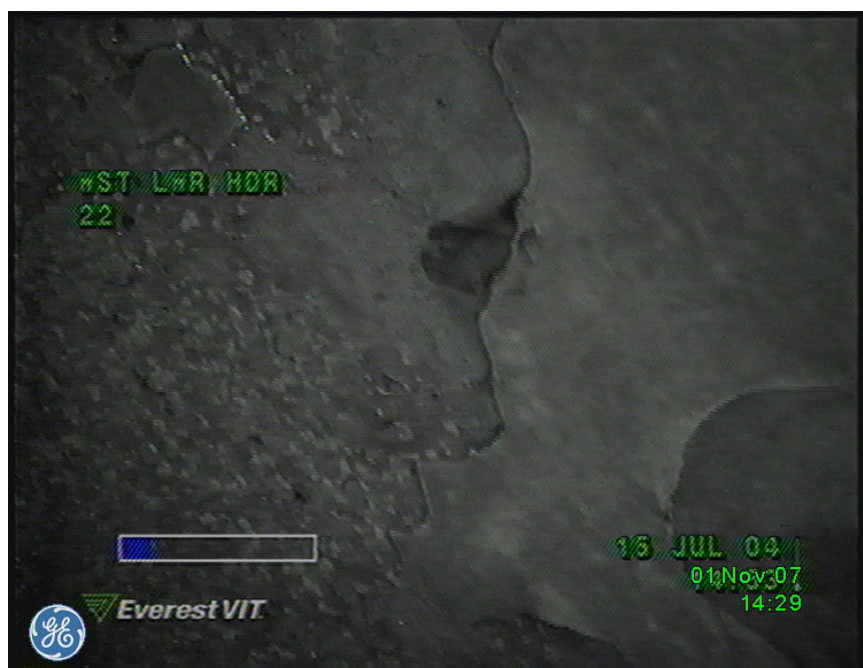
Figure 7-7 An Additional RVI Image of Low-Temperature Rust and Debris in the Lower Economizer Header That Can Be Used in a Follow-Up Evaluation by a Water Treatment Specialist
