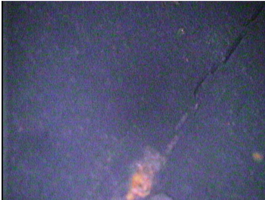
Figure 5-5 Close-Up Image of Red Rust from a Longitudinal Crack Found in the Tube (Cracks may have been present or opened more during a recent shutdown.)
