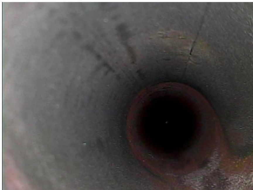
Figure 9-3 Flow-Accelerated Corrosion as Found by RVI in a Boiler Tube: This Type of Damage May Be Confirmed by External Ultrasonic Examination
