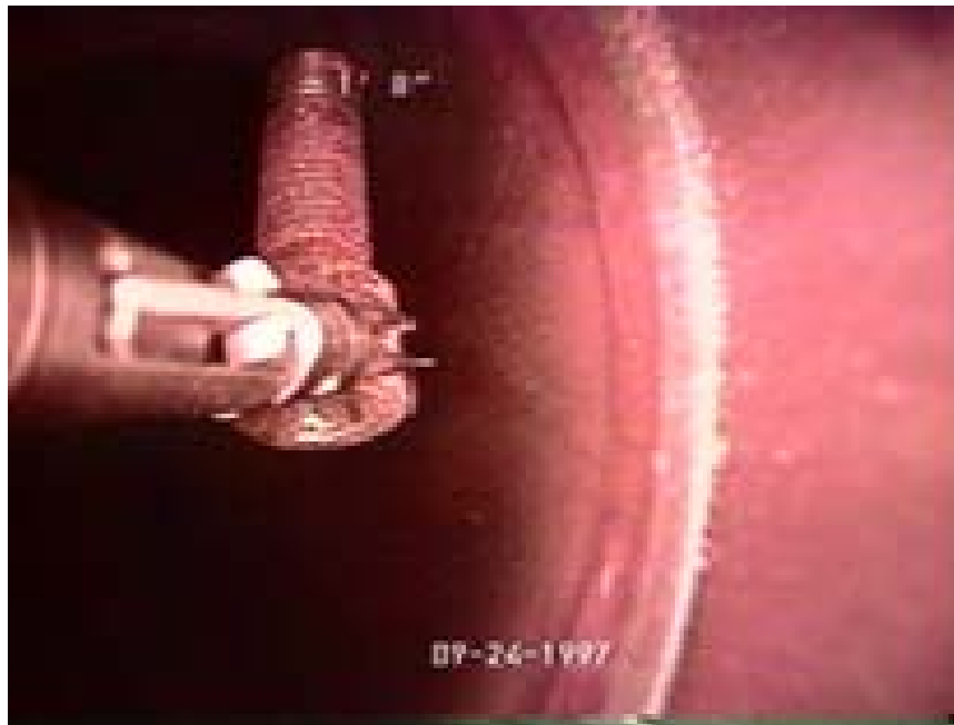
Figure 11-3 Removal of a Bolt with the Use of a Claw (Loose parts could cause tube obstruction or other impact damage.)
