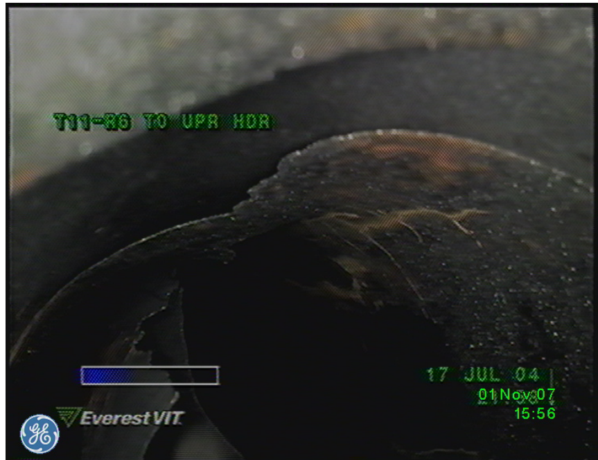
Figure 7-3 Close-Up Image of the Upper Economizer with Significant Surface Deposit (RVI should be reviewed with a water treatment specialist for additional evaluation.)
