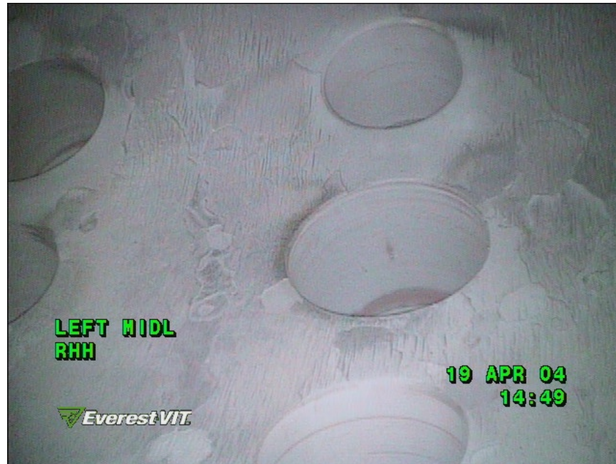
Figure 3-5 Oxide Layer on the Header Wall Is Indicative of High-Temperature Service
