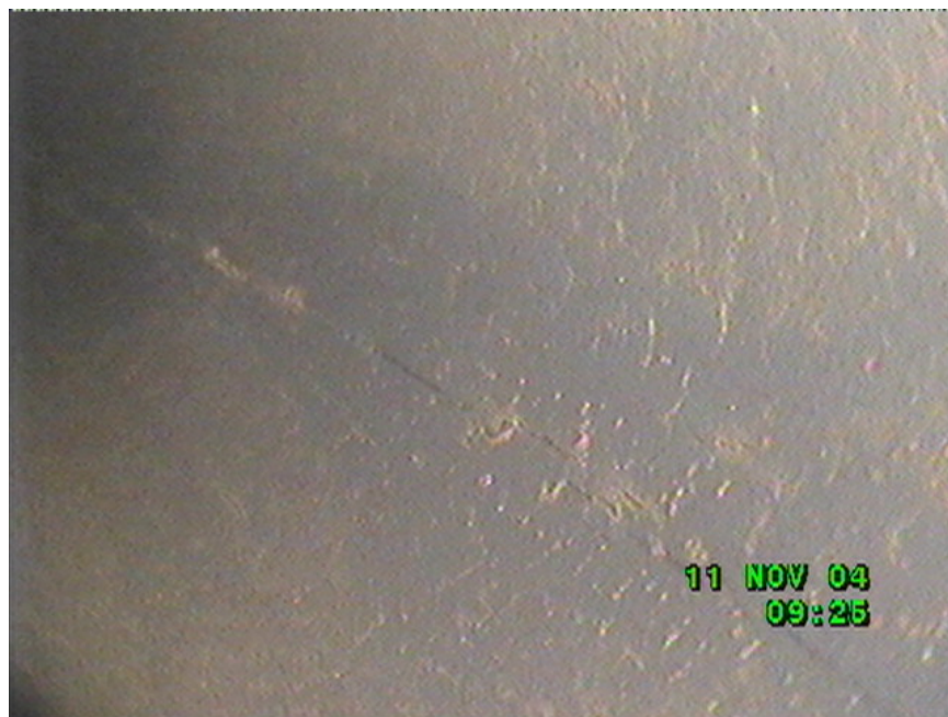
Figure 5-2 Longitudinal Crack in an Economizer Tube (Cracks are noted by dark linear indications on the remote visual inspection image.)
