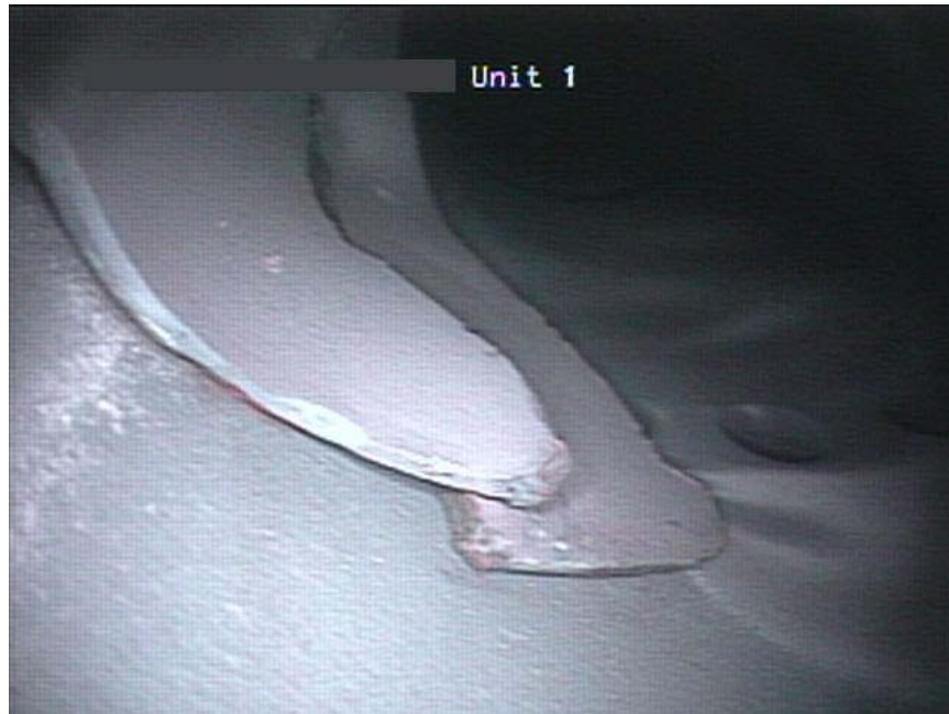
Figure 3-8 Debris in a Header May Lead to Localized Flow Disruption in the Tube and Subsequent Overheating
