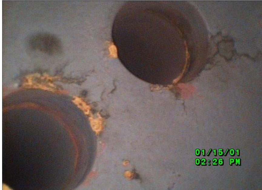
Figure 3-15 Lower Temperature Rust on Potential Cracks Can Be Identified by a Characteristic Reddish Color Using RVI
