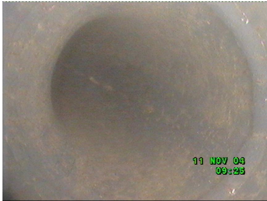
Figure 5-1 RVI Image of a “Good” Economizer Tube Two Weeks After Shutdown (The tube has a “normal” coating of high-temperature oxide.)
