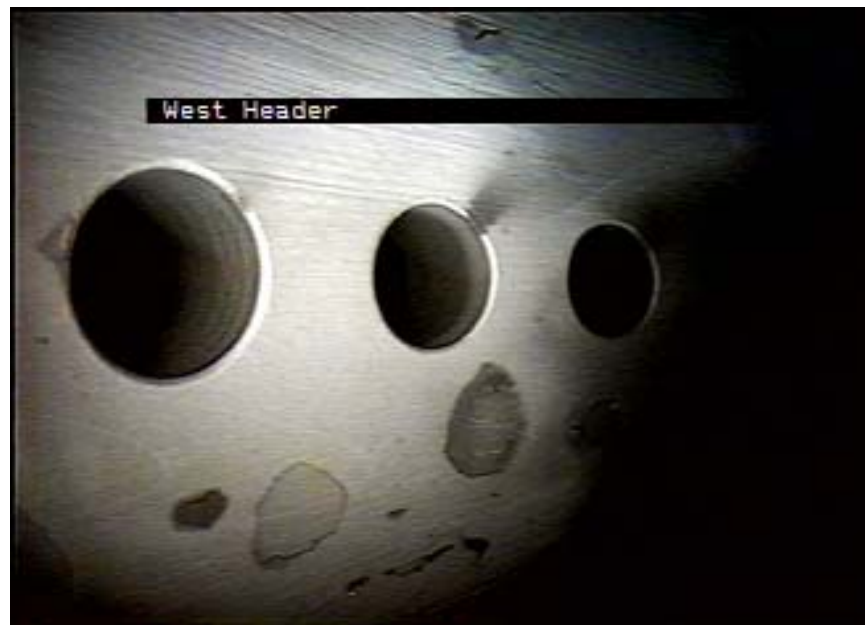
Figure 3-14 Header Penetrations with No Cracking as Documented by RVI
