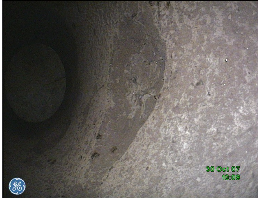
Figure 6-6 RVI Image of a Pitted Region with Hydrogen Damage (This region was subsequently removed for laboratory examination.)
