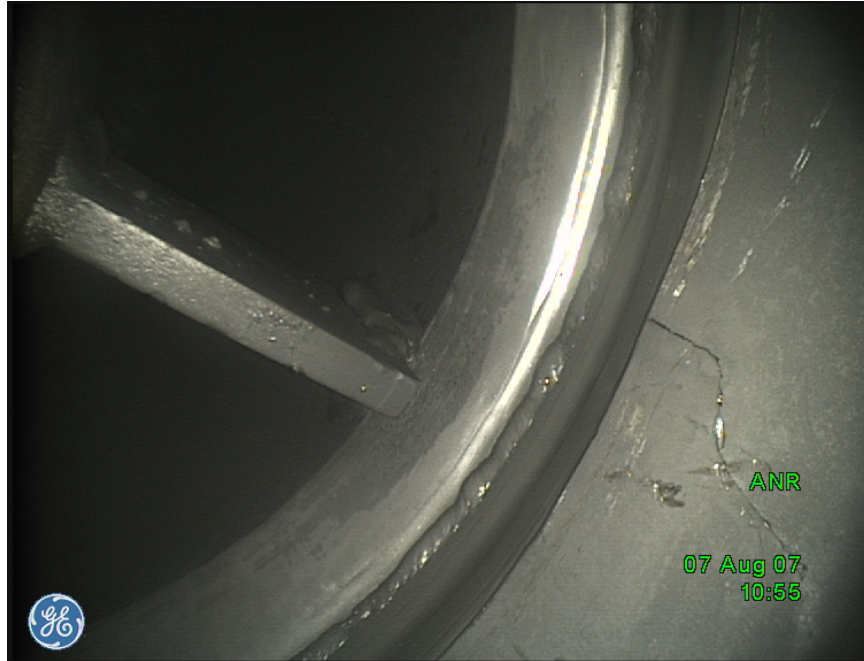
Figure 4-5 Crack in a Liner near the Nozzle (Cracks may progress by vibration and cause additional damage downstream.)
