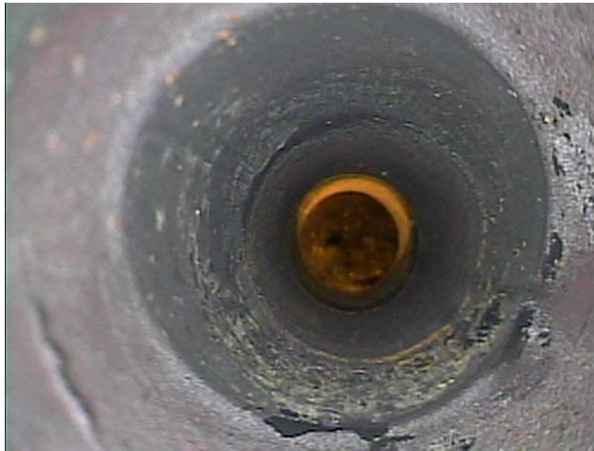
Figure 9-1 Flow-Accelerated Corrosion as Found by RVI in a Boiler Tube: Localized Wall Loss May Compromise Tube Integrity
