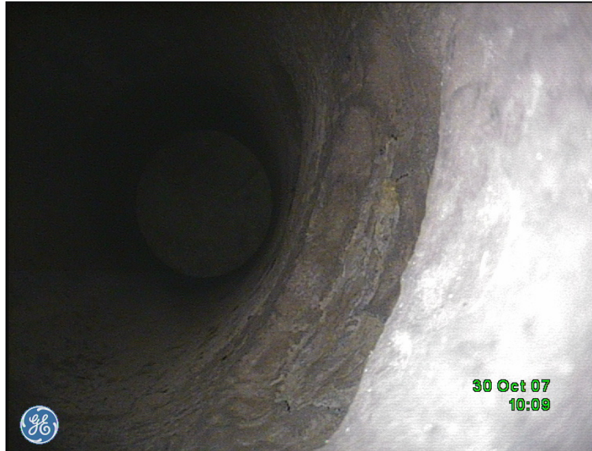
Figure 6-4 Additional RVI Image of the Pitted Region Seen in Figure 6-1 (Actual penetration depth can be confirmed by ultrasonic examination.)
