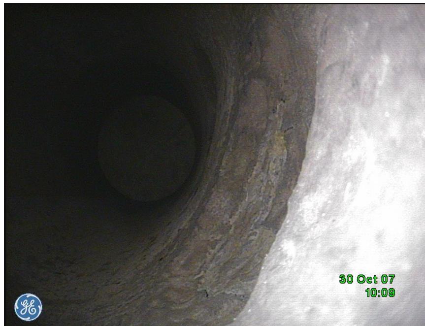
Figure 6-5 Layered Deposit on a Pitted Region (Such deposit may confirm external ultrasonic examination or identify areas for external ultrasonic examination.)
