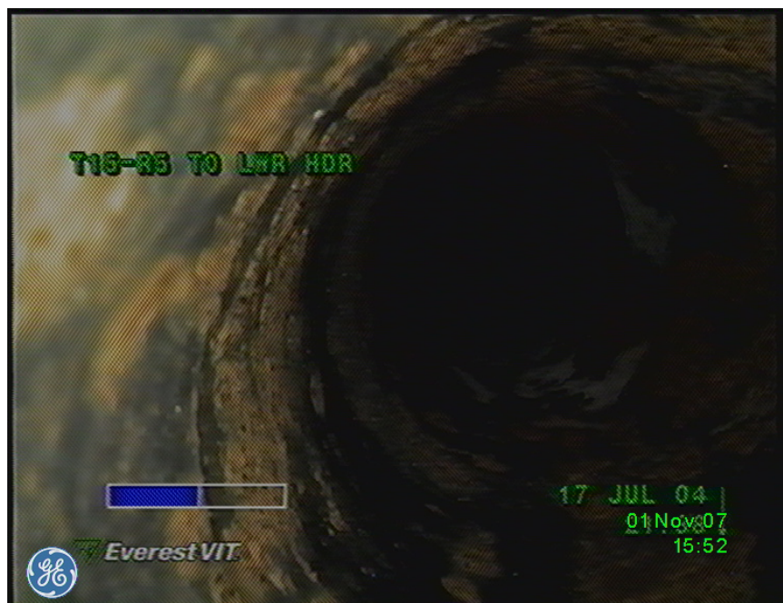
Figure 7-6 Low-Temperature Rust and Debris in the Lower Economizer Header Which Should Prompt an Evaluation of the Need for Chemical Cleaning
