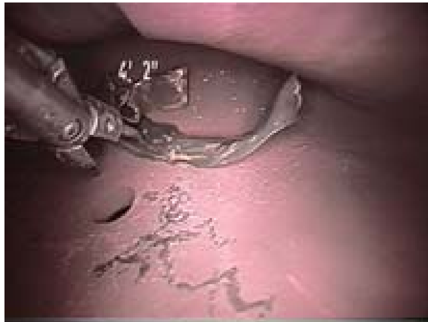
Figure 11-5 Removal of a Piece of Metal from a Boiler Feed Pump (Foreign object damage can cause significant damage in rotating equipment.)
