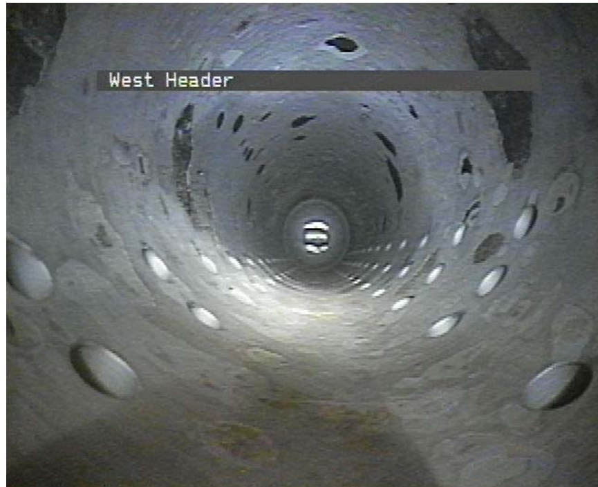
Figure 3-13 Overview of Header Penetrations with Some Spalling of High-Temperature Oxide
