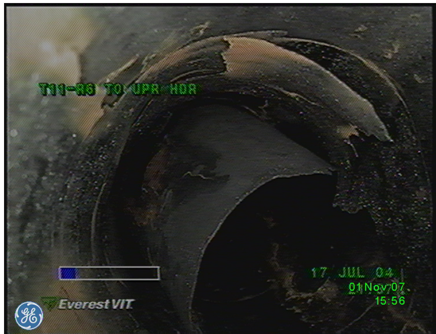
Figure 7-4 Layered Spalling in the Upper Economizer with Surface Deposit (This amount of deposit could be considered excessive and should be further evaluated.)
