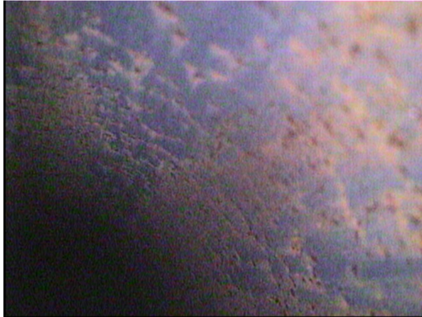
Figure 5-3 Crazed “Mud-Cracking” Type of Damage Found on the Inner Surface of an Economizer Tube
