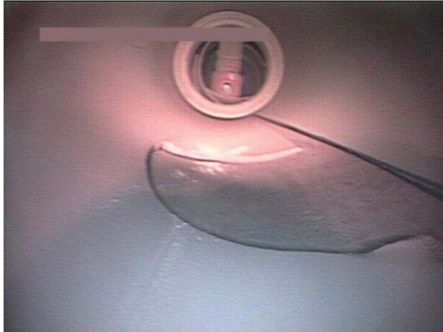
Figure 4-2 Missing Liner Section in a Desuperheater (Fragments from this liner can be seen in Figure 4-1.)
