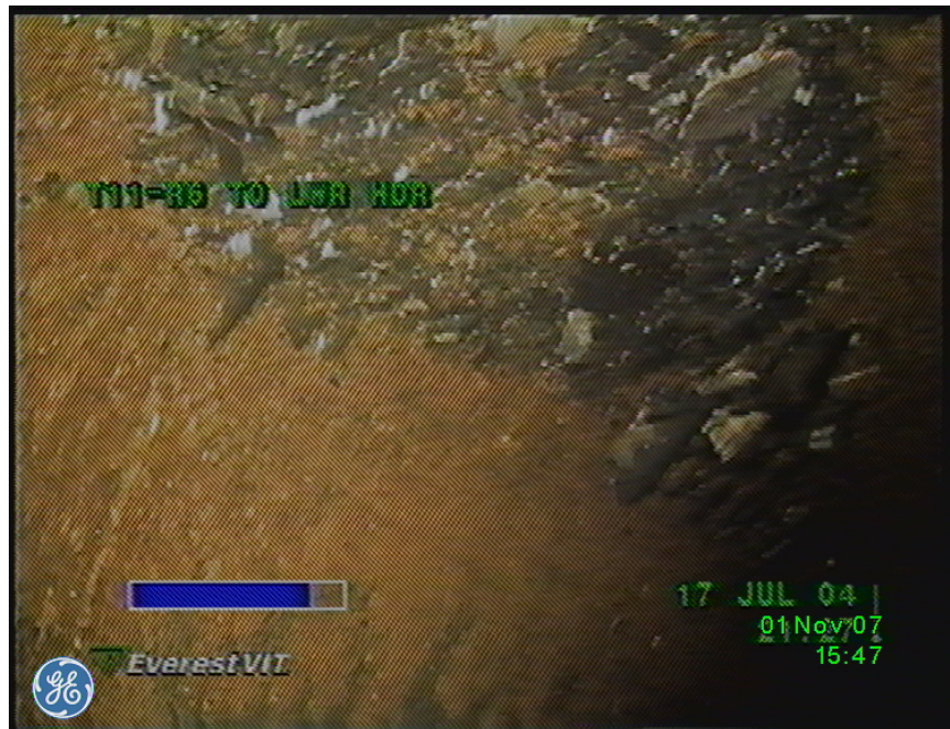
Figure 7-5 Lower Economizer Header with Some Accumulation of Low-Temperature Rust (This may be a result of inadequate blowdown practices.)
