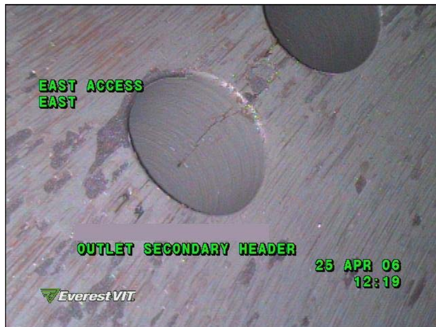
Figure 3-6 Oxide Layer on the Header Wall, with Some Isolated Spalling, Is Indicative of High-Temperature Service
