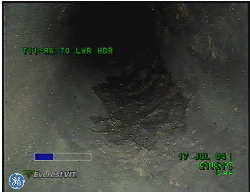
Figure 7-8 RVI Image of High-Temperature Scale and Debris in the Lower Economizer Header That Can Be Used for an Evaluation by On-Site or Corporate Specialists
