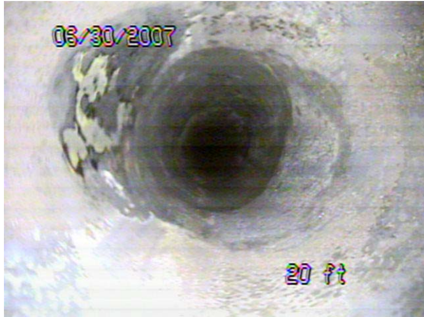
Figure 9-4 Flow-Accelerated Corrosion as Found by RVI in a Boiler Tube: Tube May Require Removal for Additional Laboratory Evaluation
