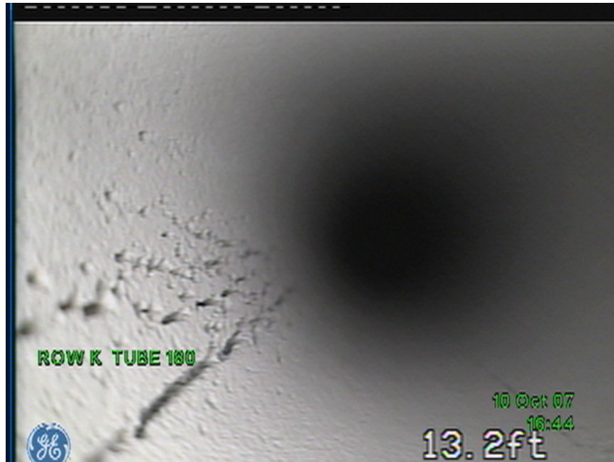
Figure 10-6 Corrosion Fatigue Cracking in a Boiler Tube with Multiple Longitudinal Cracks
