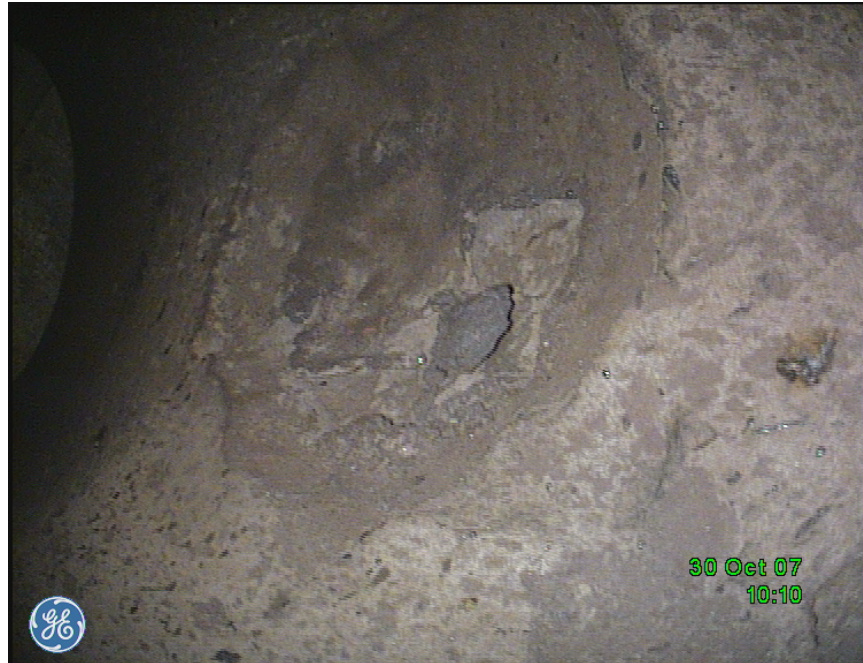
Figure 6-1 Inner Surface Deposit with a Pit as Found by RVI (This type of deposit and subsequent pitting may be indicative of hydrogen damage in waterwall tubes.)
