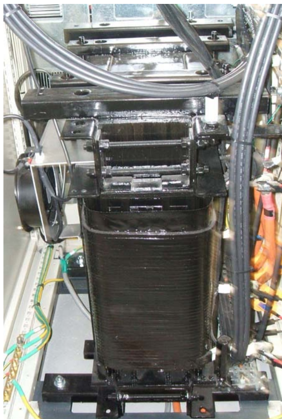
Figure 1-6 Series Injection Transformer of the AVC-Store
