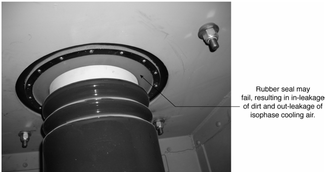
Figure 12-9 24-kV Generator Bushing with a Rubber Seal
