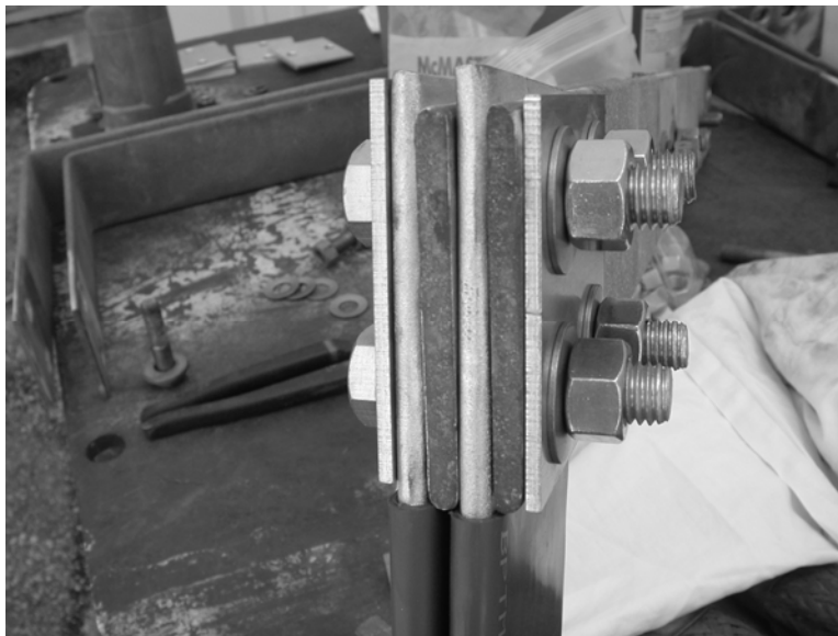
Figure A-4 Improved Connection with Stainless Steel Plates on the Outside of the Bus Bars to Spread the Compressive Load of the Bolts, Stainless Steel Bolts, and Belleville Washers
