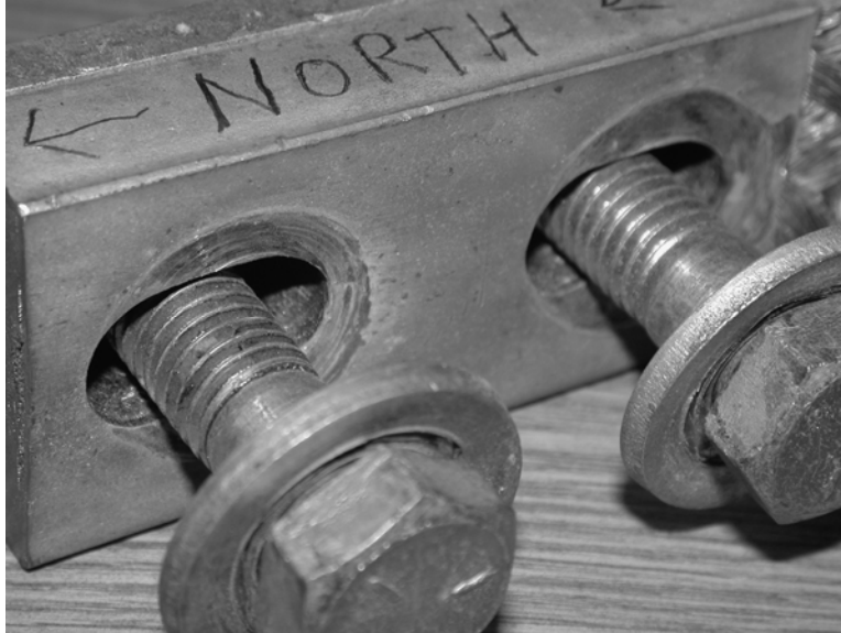
Figure A-5 Flexible Strap Ends That Have Been Overtorqued into Concave Condition
