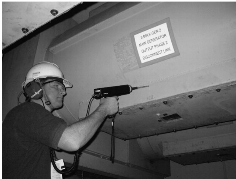
Figure 11-7 Proper Technique for Monitoring Isophase Bus with an Acoustic Contact Probe
