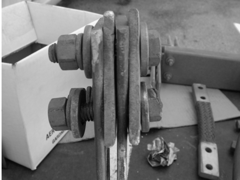
Figure A-3 Typical As-Found Bolted Bus Bar Connection Using Steel Bolts and Flat Washers
