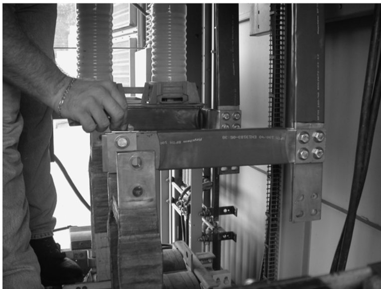
Figure A-2 Improved Neutral Connection Using Stainless Steel Plates on Both Sides of the Bus Bar, Stainless Steel Bolting, and Belleville Washers (The electrician is making a cursory examination of the connection point with a 0.002-in. [0.051-mm] feeler gauge.)
