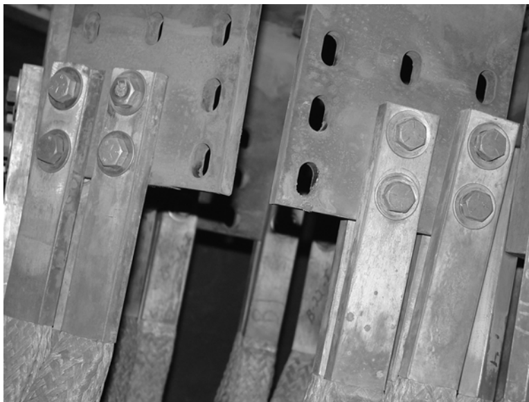
Figure A-10 Typical Main Lead Connection Plate to Isophase Bus Work Flexible Links
