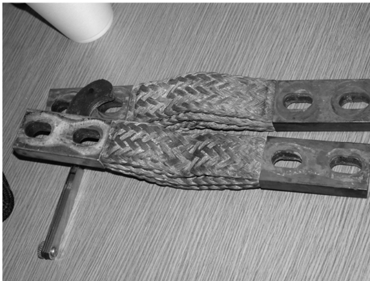
Figure A-6 Typical Electrical Connection Pattern on Flexible Strap Ends; Design Is for the Entire Surface to Be in Contact with the Bus or Neutral Bus Segment (Poor electrical connections have caused the bus and the strap ends to be heated.)
