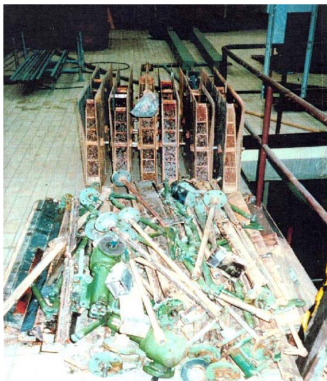
Figure 6-5 Obsolete Parts Removed from HE-2 Strainers
