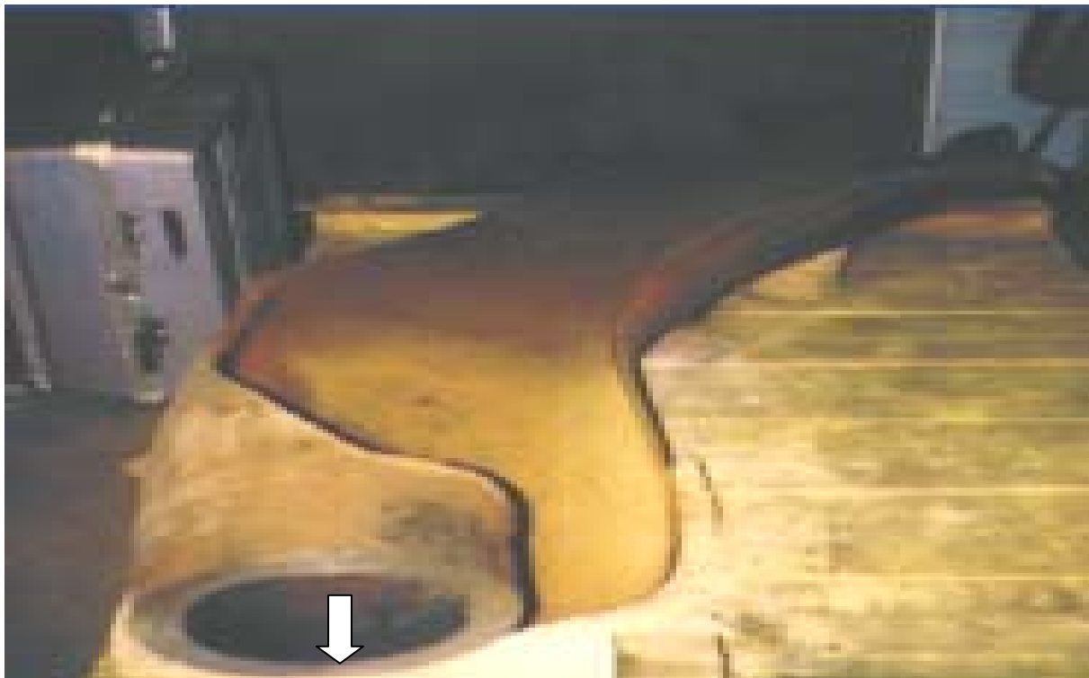
Figure 3-11 Pleasant Prairie Power Plant Feedwater Pipe (Photograph courtesy of Wisconsin Electric)
