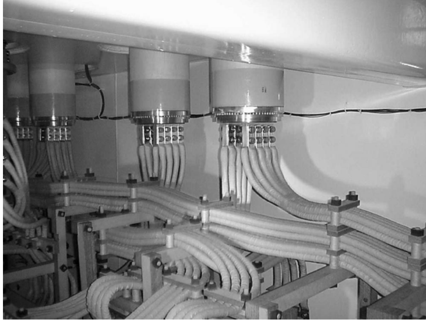
Figure A-22 Flexible Connections Between Transformer Winding and Bushings Courtesy of Exelon
