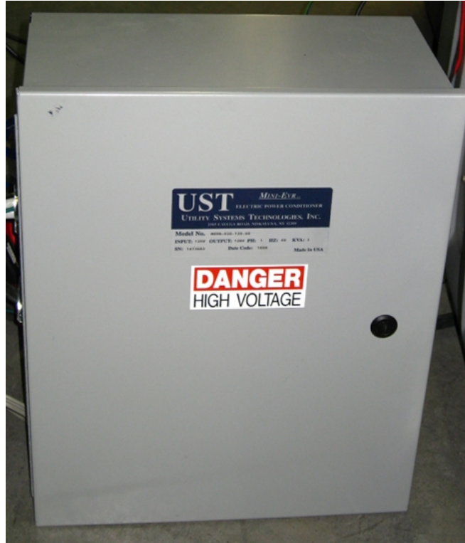
Figure 1-1 Photograph of the 3kVA Mini-EVR™ From Utility Systems Technologies, Inc.
