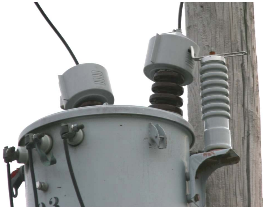
Figure 3-8 It is Unlikely that this Arrester is providing Adequate Protection Given the Length of the Spark Gap
