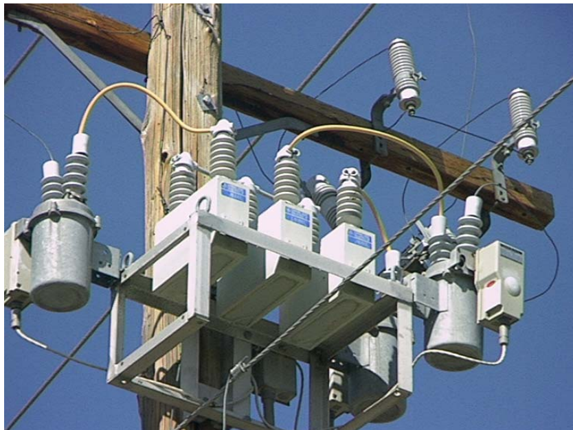
Figure 3-12 Capacitor Bank with Factory-Installed Wildlife Guards
