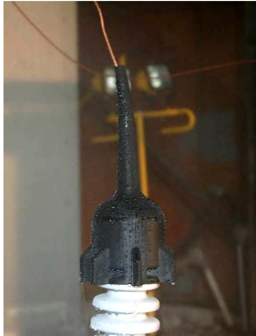
Figure A-7 Wildlife Guard from Sample Set L Installed on a Test Fixture
