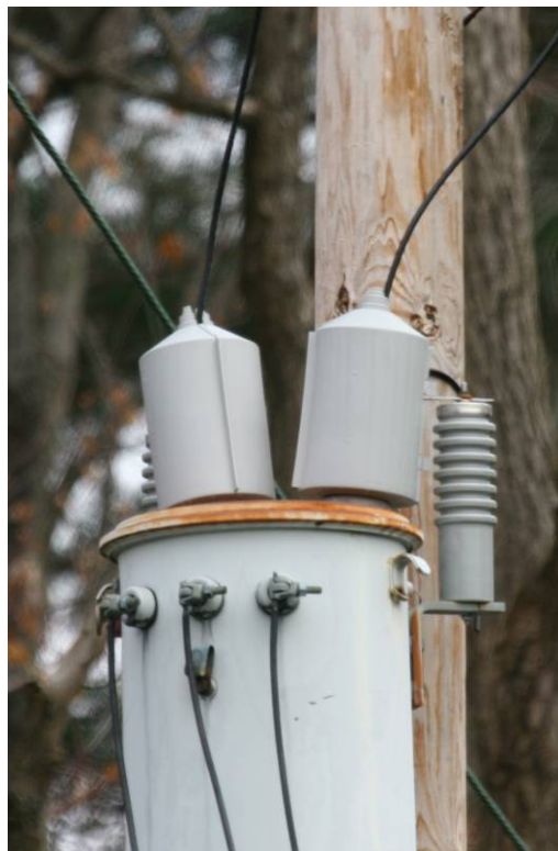
Figure 3-3 Example of Improperly Installed Bushing Covers
