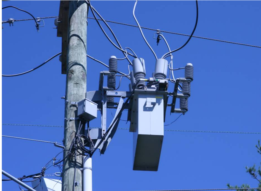
Figure 3-11 Wildlife Guard Application for Reclosers – Bushing Covers, Arrester Caps, Covered Leads, and Non-Conductive Brackets
