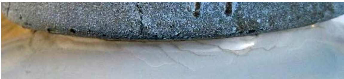
Figure 2-5 Close-Up View of Cracks Just Below the Energized Trunnion Cap of Sample #2
