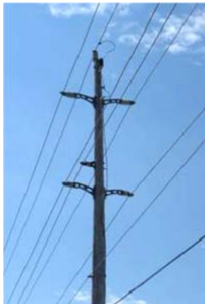
Figure 1-1 Example of the Armless Construction Design Employed on the We Energies Distribution System
