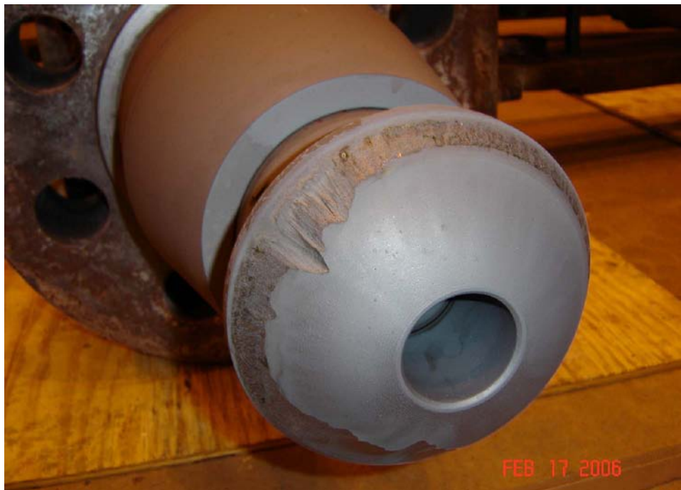
Figure 5-8 Solid particle erosion damage in control valve disc 2 (Courtesy of TVA)
