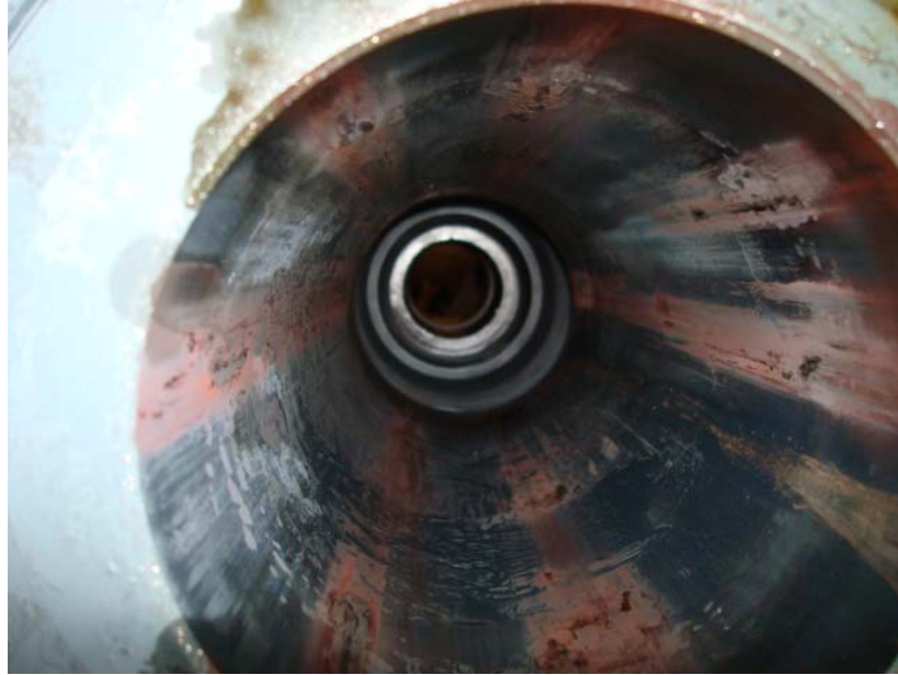
Figure 3-3 Nitrided 422 stainless steel bushing after 48,000 hours service with thick oxide scale
