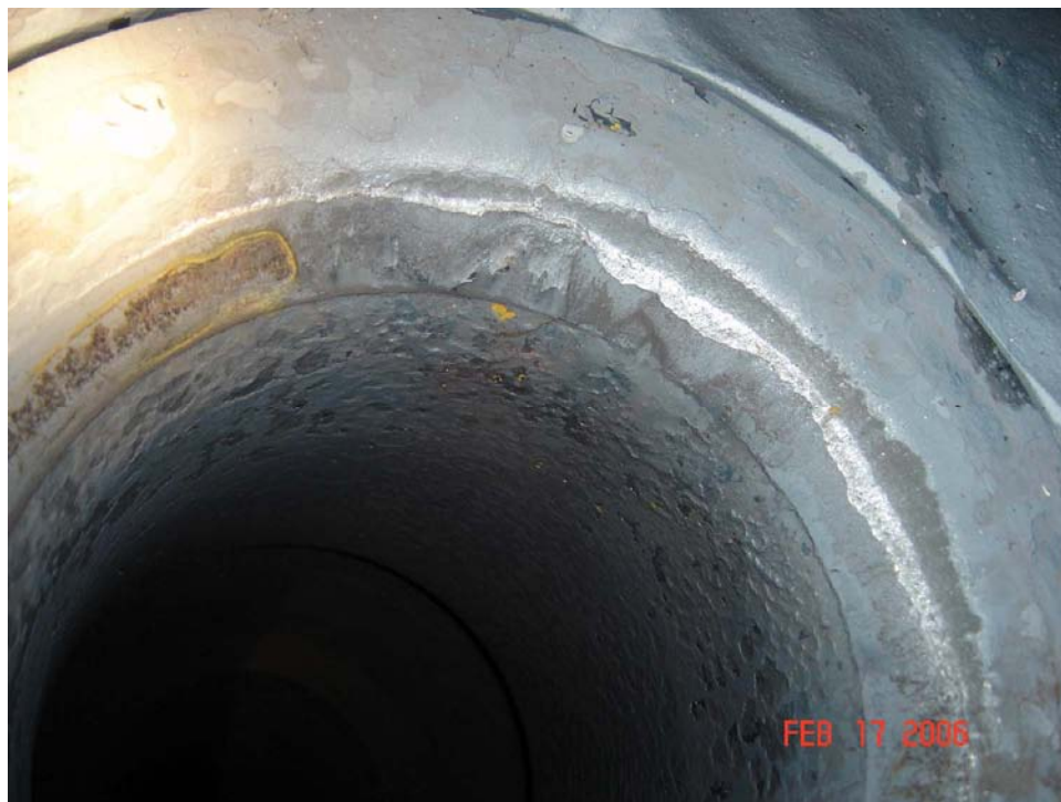
Figure 4-6 Detailed view of solid particle erosion in the seat of control valve 1
