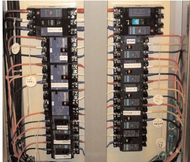
Figure 16. Metal Etch Loader: Power Feed Circuit Breaker (from Metal Etch Distribution Panel)
