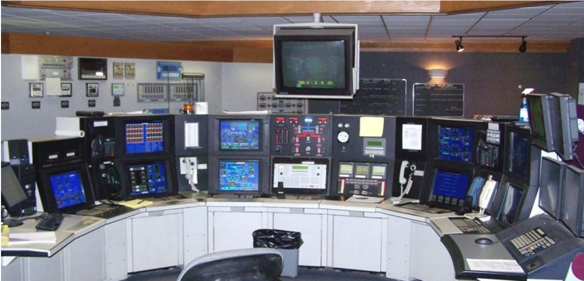
Figure 2-1 GGS Unit 2 Control Room Console
