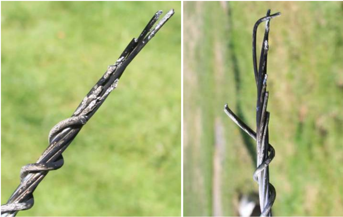
Figure 4-16 The End of the Conductor That Becomes De-Energized After Separation Shows That the Conductor Strands Separate at Different Locations
