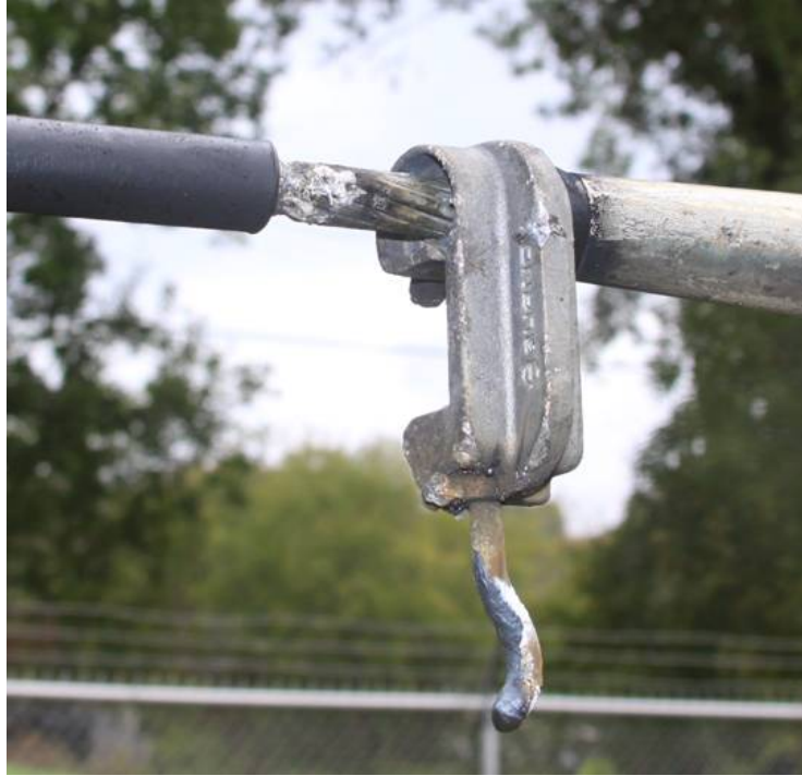
Figure 4-31 This Improperly Installed APD Allowed Significant Damage to the Conductor
