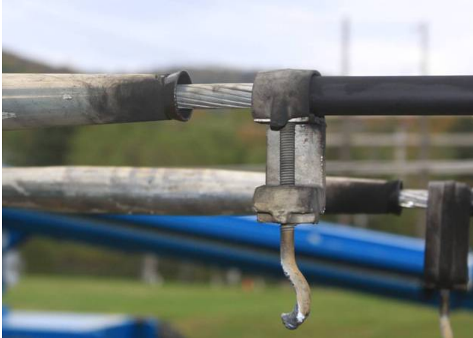
Figure 4-29 This Arc Protective Device Prevented the Conductor from Being Damaged During the Arcing Fault
