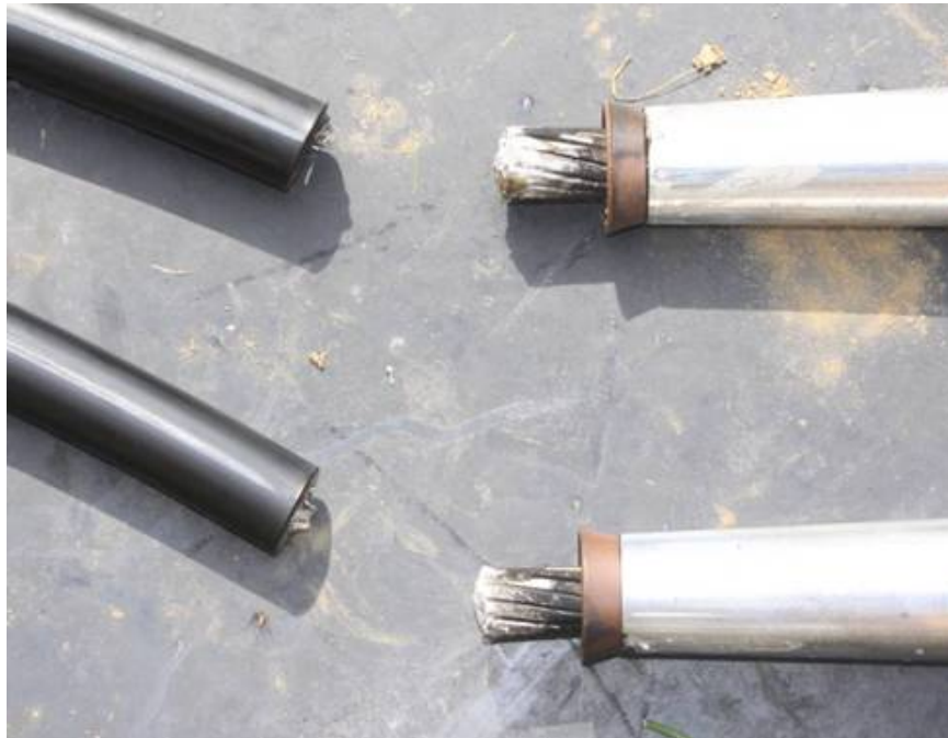
Figure 4-27 Breakage Occurred on the Load Side of the Automatic Splices
