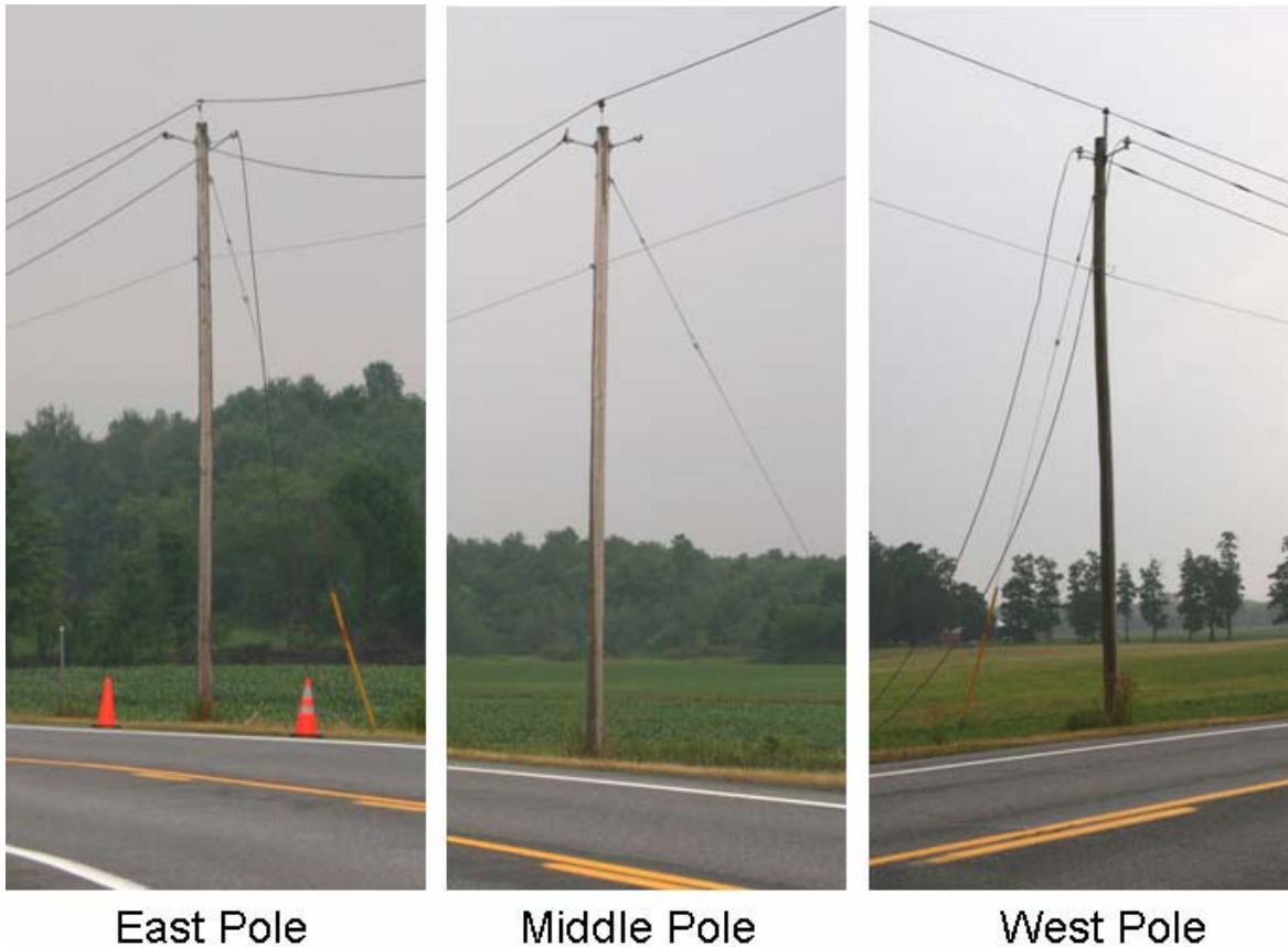
Figure 1-1 A Lightning-Induced Burndown Event on Covered Conductors Affecting the Conductor over Two Pole Spans
