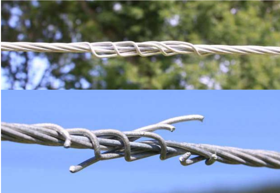
Figure 4-23 Conductor “Bird Caging” Due to a Motoring Arc Lingering at These Locations
