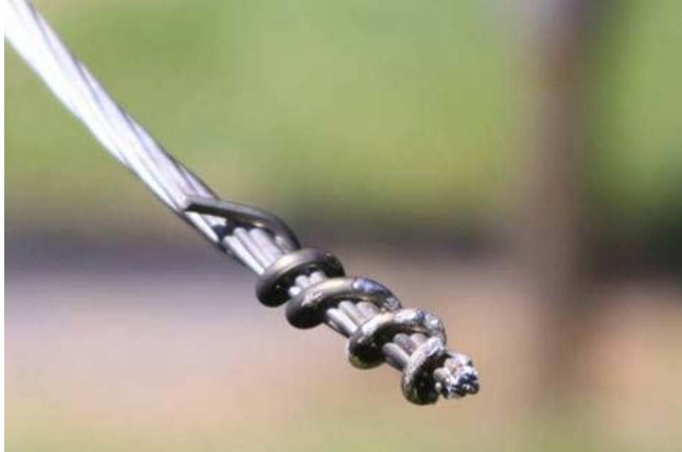
Figure 4-17 The End of the Conductor That Remains Energized After Separation Continues Arcing, Causing the Broken Strands to Be Vaporized Back to a Nub
