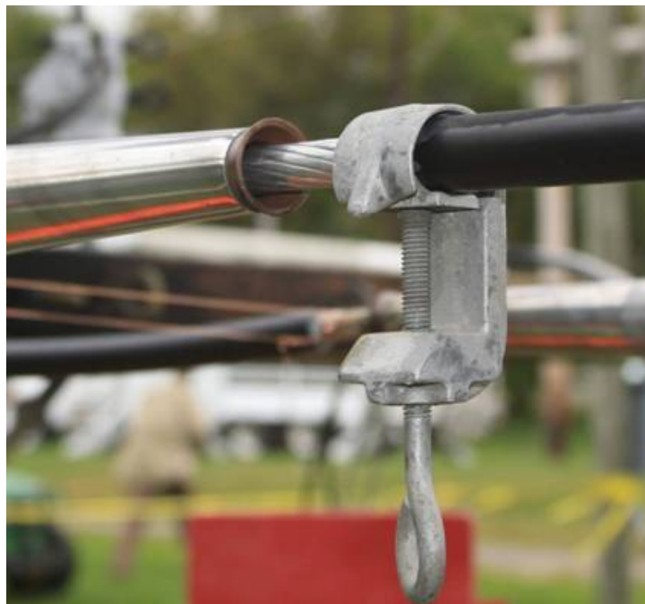
Figure 4-28 Properly Installed Arc Protective Device
