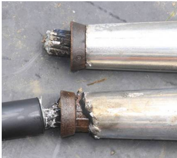
Figure 4-25 The Lower Splice and Conductor Suffered Severe Damage and Probably Would Have Broken Had the Conductor Been Under Tension
