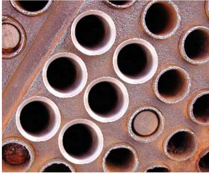
Figure 7-4 Example of a set of heat exchanger tubes with installed sleeves
