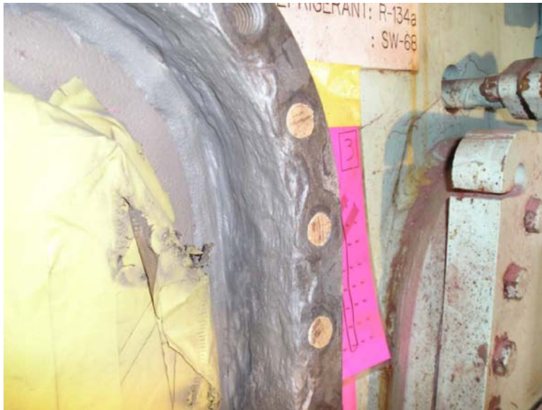
Figure 7-8 Flange condition before repair with a metal replacement epoxy
