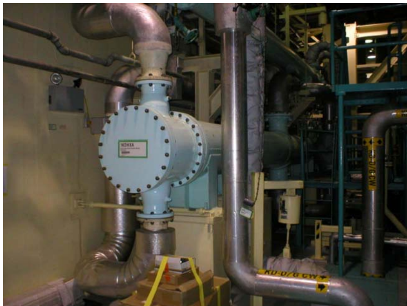
Figure 1-2 Diesel engine jacket water heat exchanger
