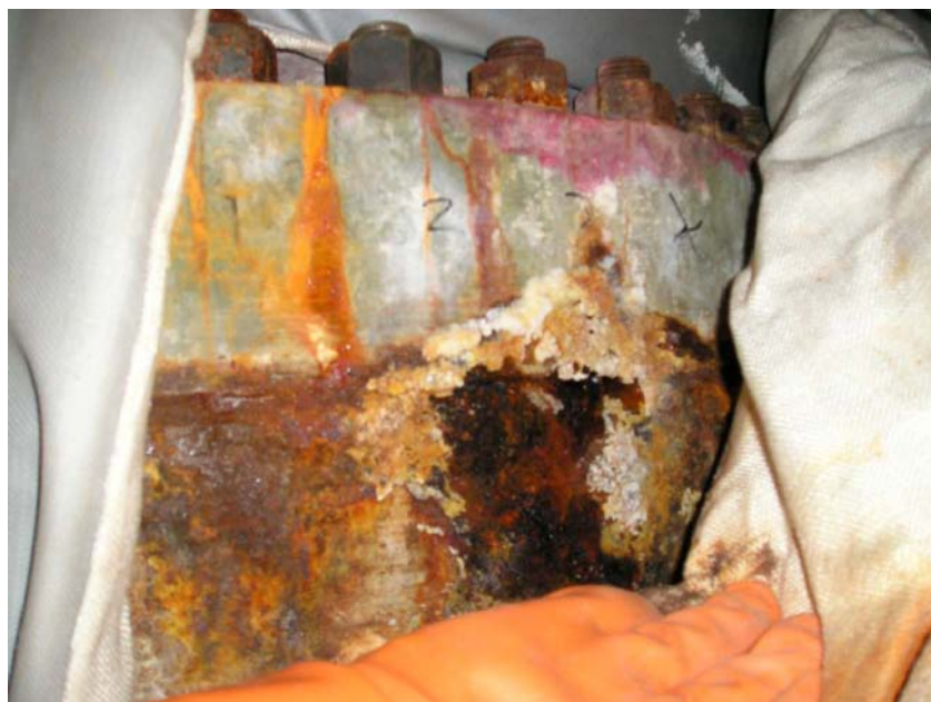
Figure 4-9 Effects of a gasket failure in a heat exchanger
