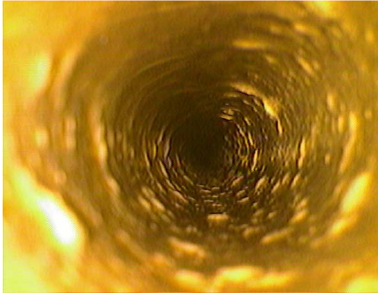
Figure 6-3 Stainless steel tube fouling before brushing
