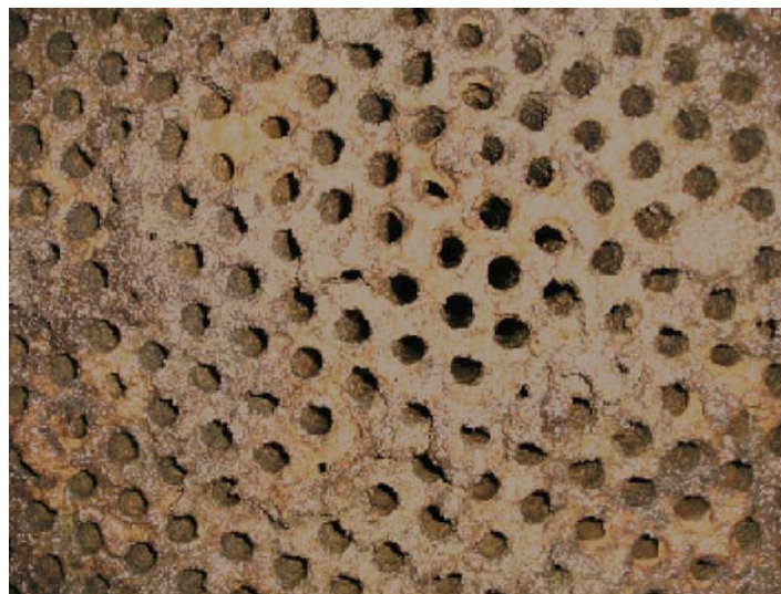
Figure 3-1 Biofilm fouling in a heat exchanger
