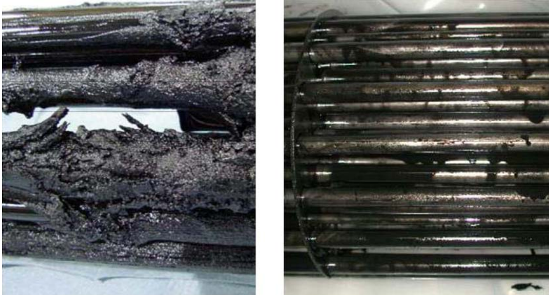
Figure 5-1 EDG heaters pre- and post-modification
