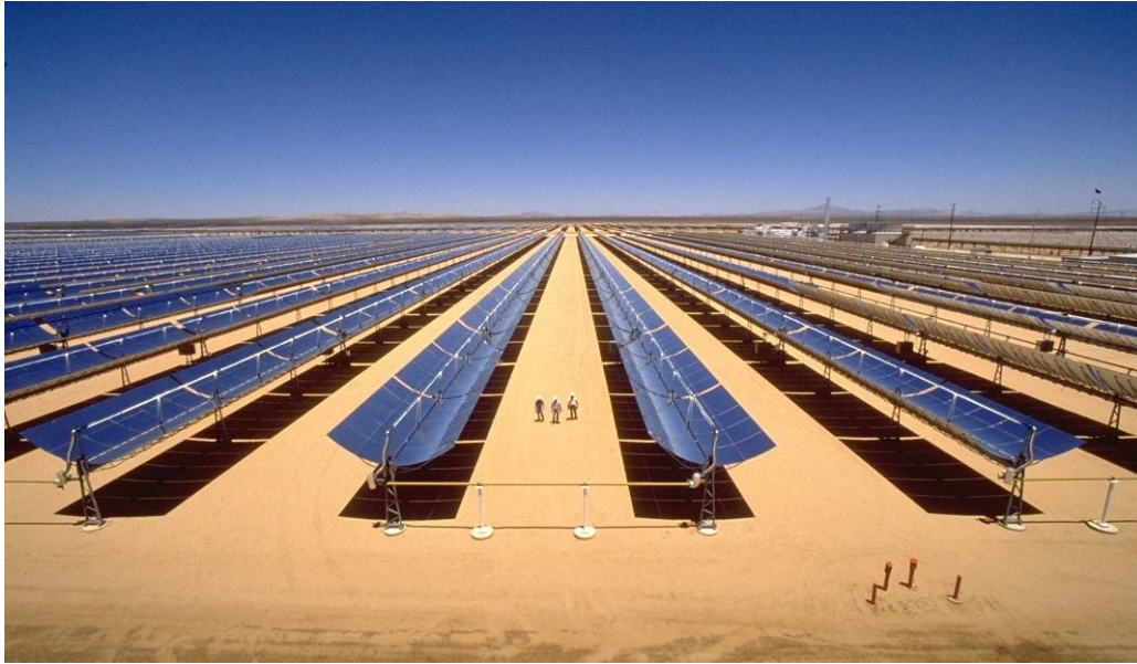
Figure 2-1 Parabolic Trough Collector Field
