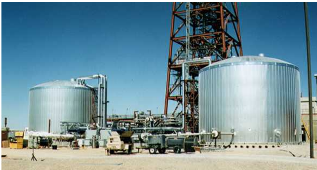
Figure 2-10 Thermal Energy Storage System at Solar Two, Barstow, CA
